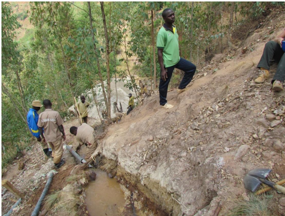
Figure 23: Water and tailings discharge to valley
