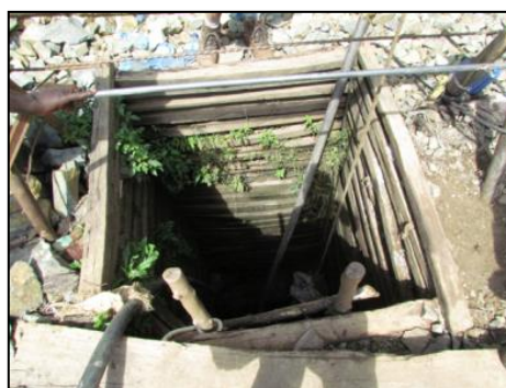
Figure 13: Although well-timbered, this shaft is plagued by frequent flooding and is at a depth prone to collapse
