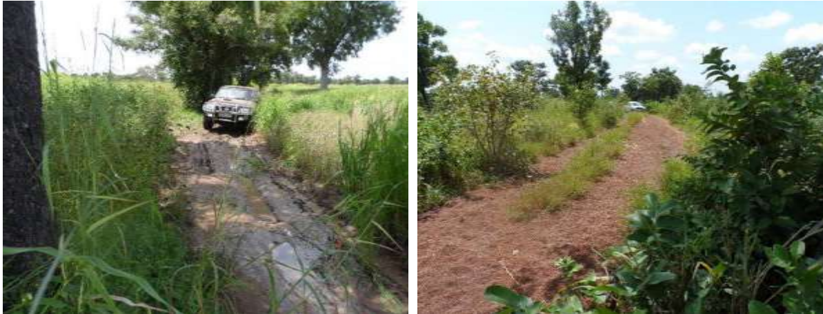
Figure C.14: Localised drainage and passability problems
