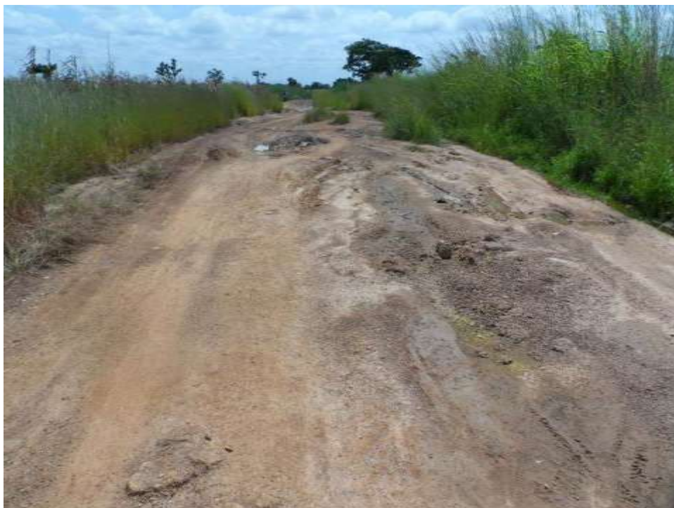
Figure C.7: Poorly drained area with weak silty material
