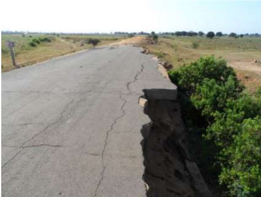
Figure B.8: Damage to embankment and loss of road at lowest point
