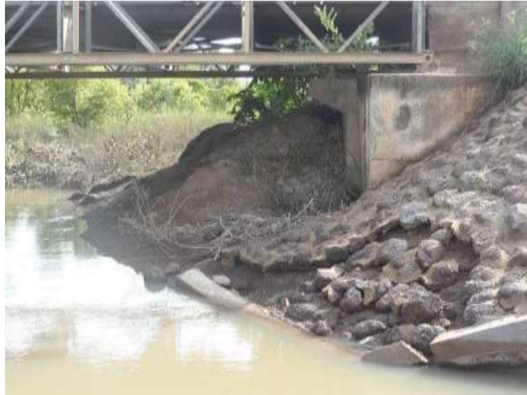
Figure C.18: Erosion of bank protection beneath Bailey Bridge
