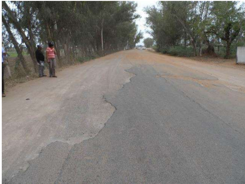
Figure 25: Loss of surfacing due to overtopping
