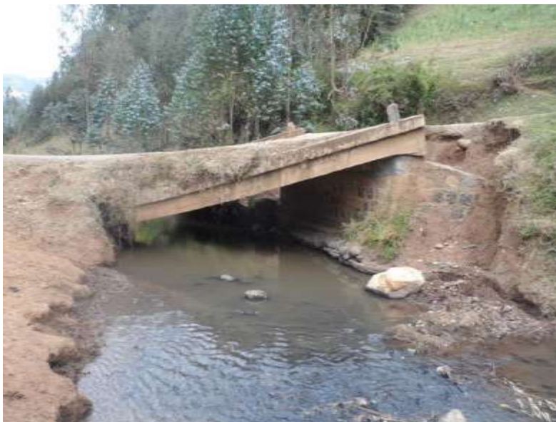
Figure A.13: Collapsed bridge at km 47.4
