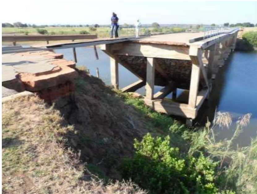
Figure B.5: Loss of bridge approach fills and collapse of one pier during 2012 flooding
