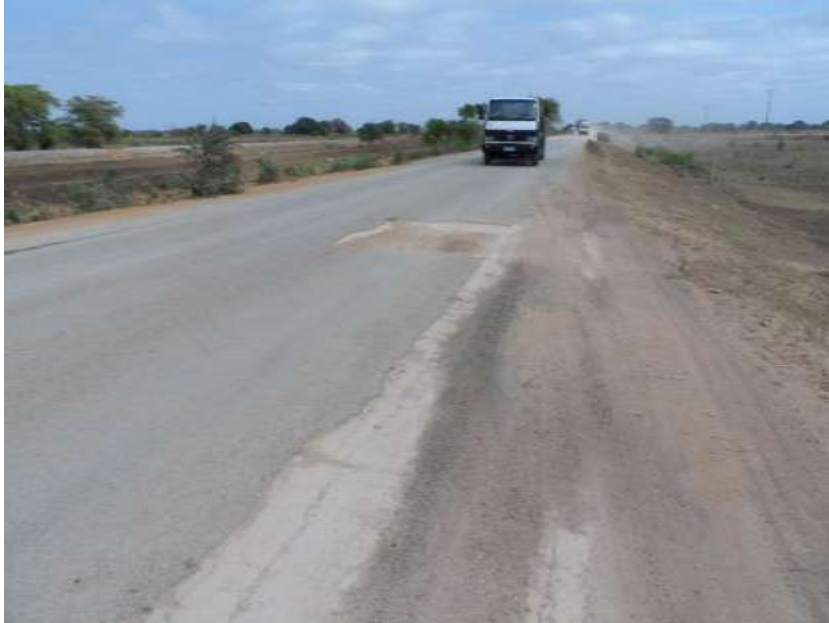
Figure B.32: Loss of seal due to water penetrating at edge of seal
