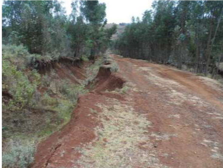
Figure A.8: Erosion alongside the road on a steep grade
