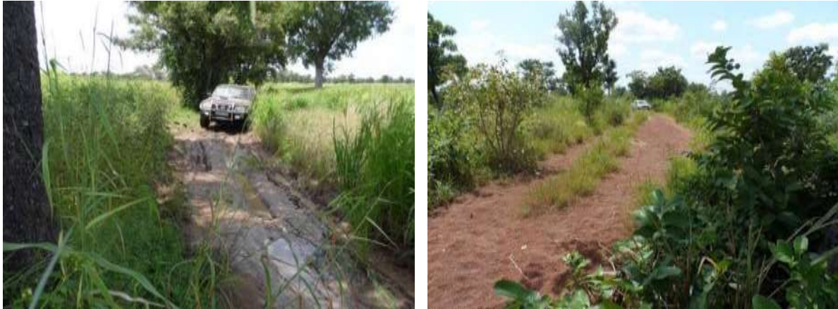
Figure 38: Existing muddy and fine gravel earth road with passability problems
