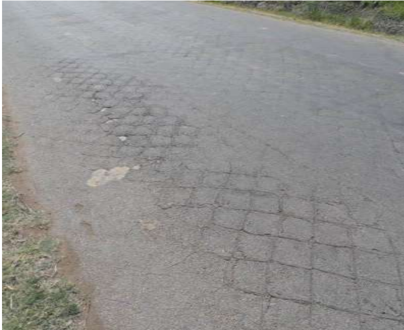
Figure B.34: Open cracks reflecting through from actual Geocell grids
