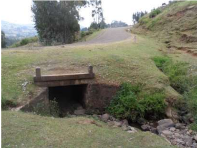
Figure A.15: Small concrete bridge with eroded inlet channels
