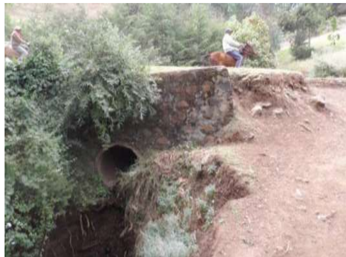
Figure 13: Erosion around, below and adjacent to culvert
