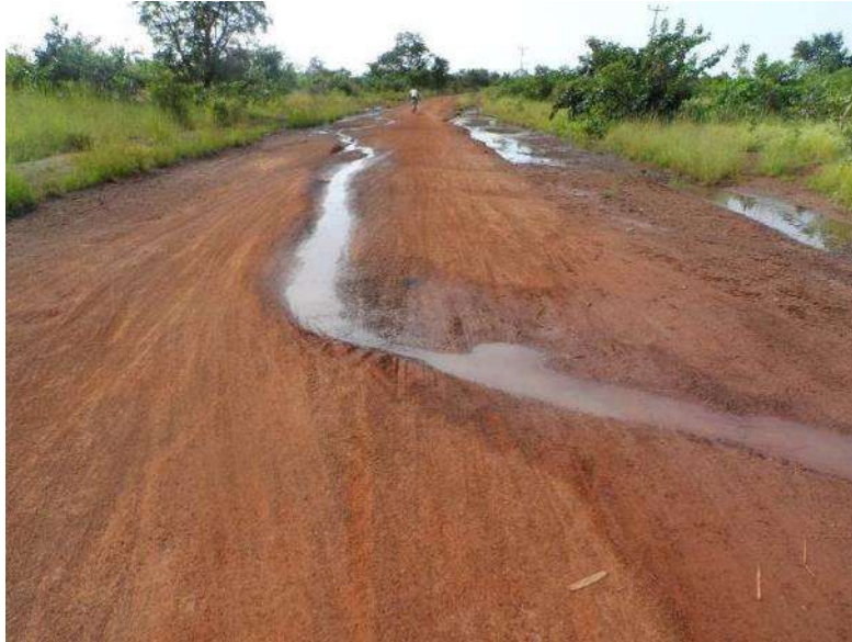
Figure C.22: Erosion of road surface and side drains
