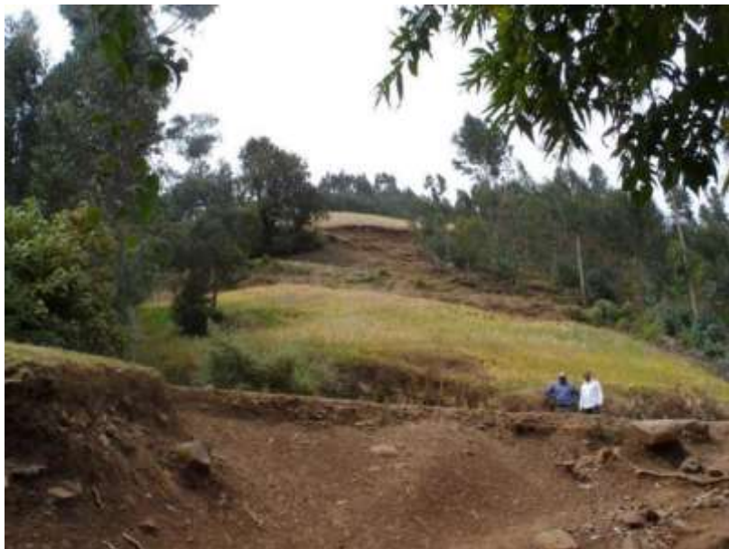
Figure A.11: Landslide scar on hill with erosion of embankment in foreground
