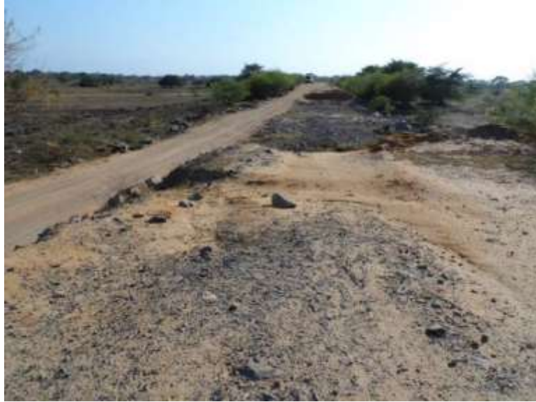
Figure B.4: Site of embankment and culvert removed by flooding with deviation on the left
