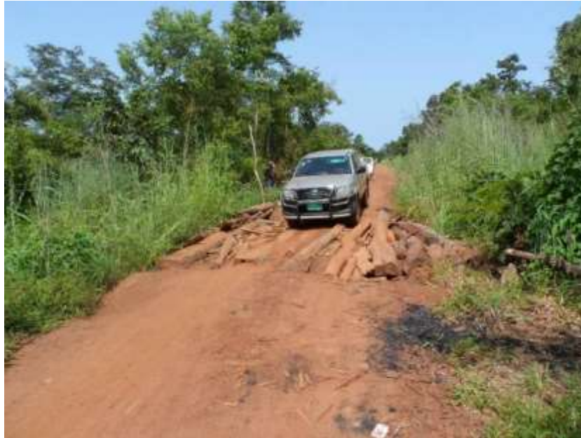
Figure C.16: Collapsed culvert repaired using logging off-cuts
