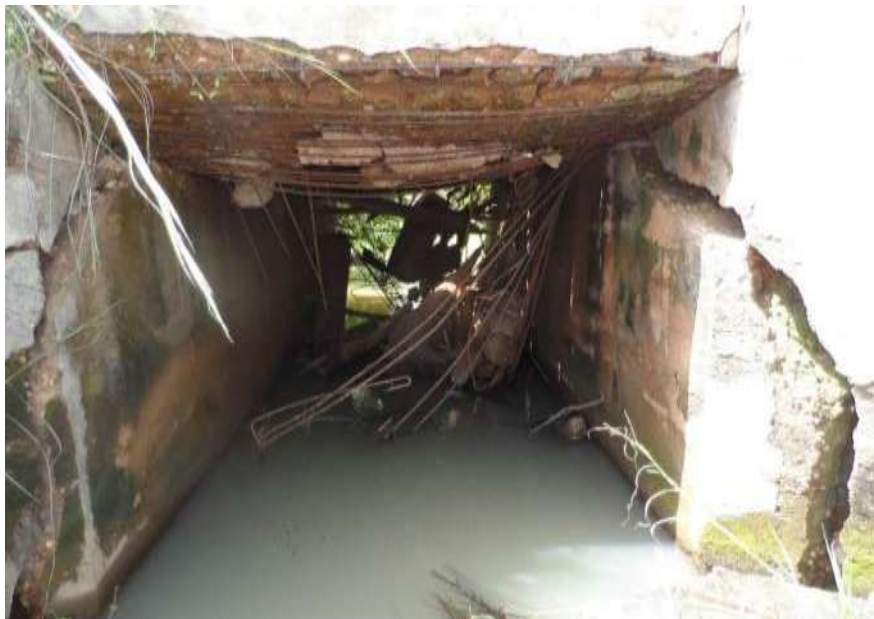
Figure C.19: Collapsed concrete bridge showing severe damage to deck, abutments and wing-walls.
