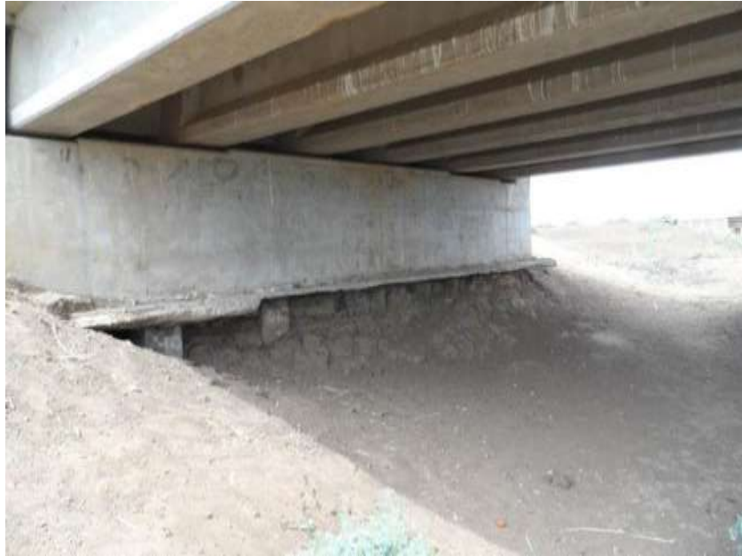
Figure B.40: Erosion of fill around abutments during flooding
