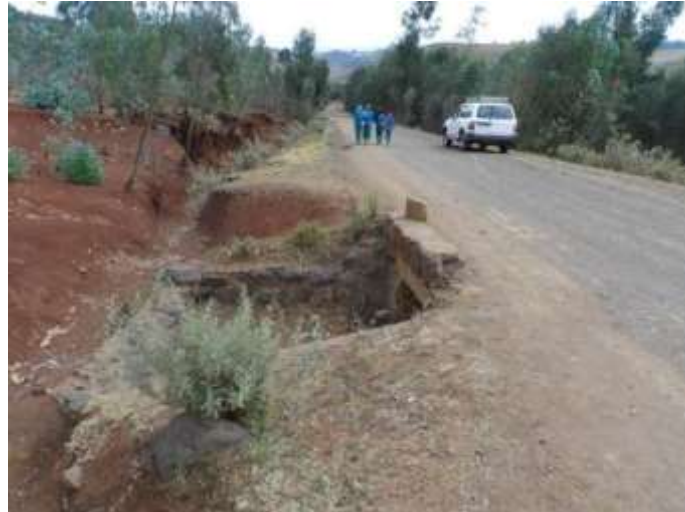
Figure 11: Erosion of shoulders and side drains on steep grade
