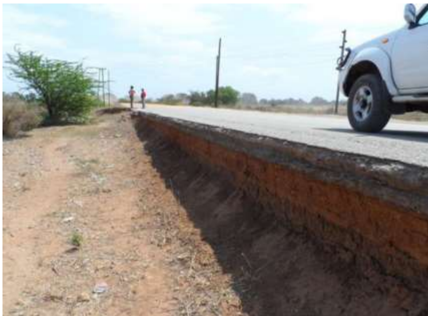
Figure 28: Erosion of embankment and undercutting of pavement caused by overtopping
