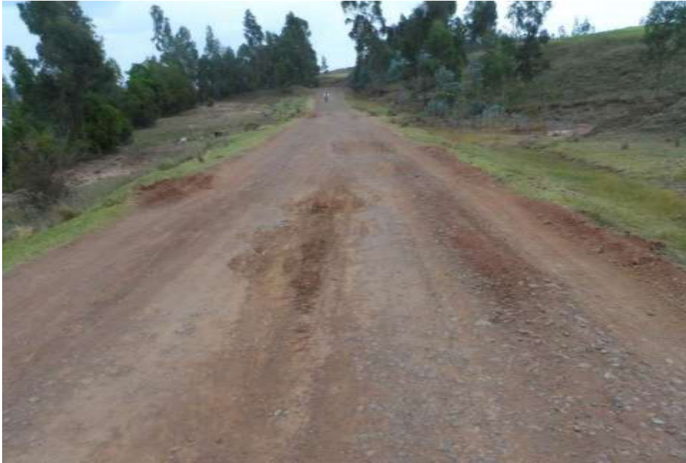
Figure A.16: Shear failures resulting from localised drainage problems
