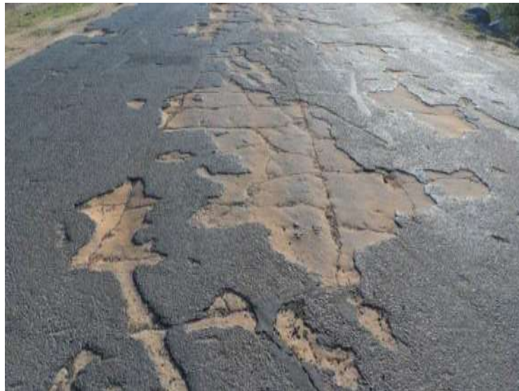
Figure B.2: loss of surfacing from cement stabilised sand base
