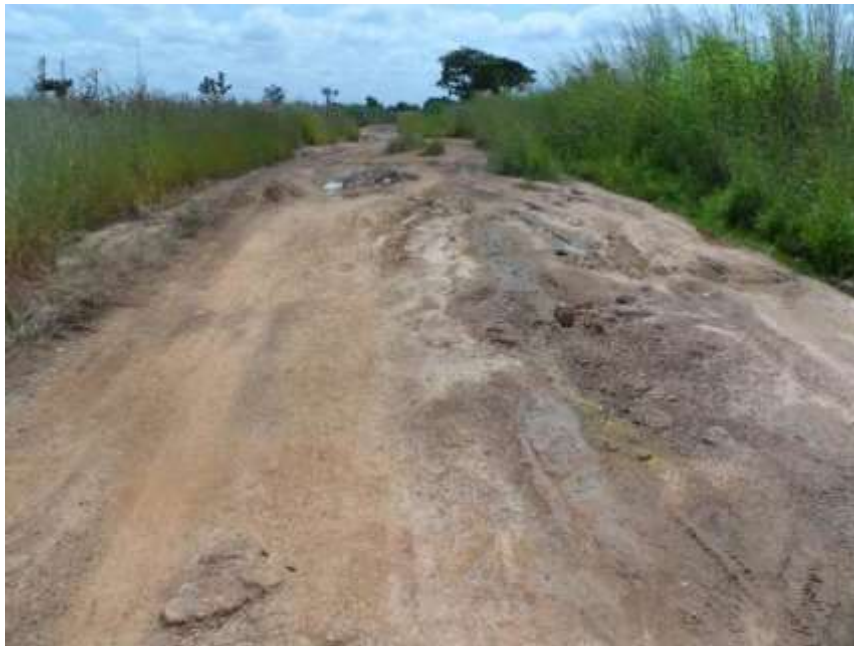
Figure 37: Eroded, poorly drained section of road with laterite outcrops
