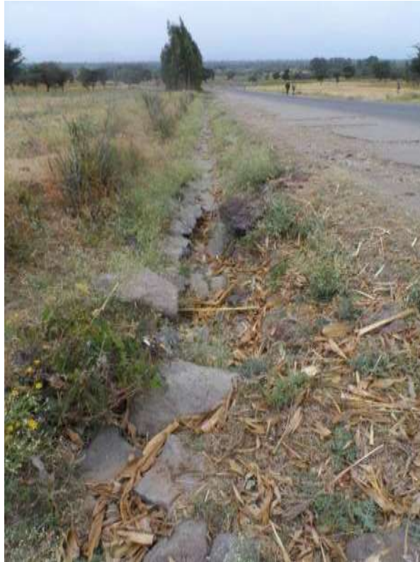
Figure A.22: Damage to mortared stone pitched side drain and continued edge-break problems
