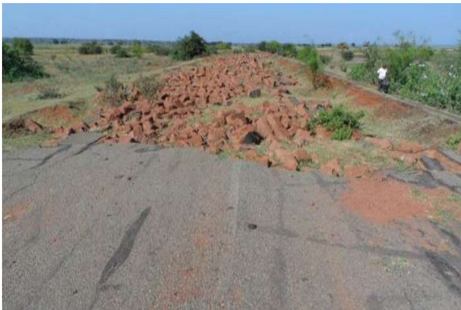
Figure B.9: Total loss of road and embankment caused by overtopping and undermining from the downstream side
