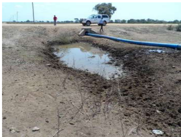
Figure B.38: Photo of 2012 flooding showing localised turbulent flow at low points in embankment
