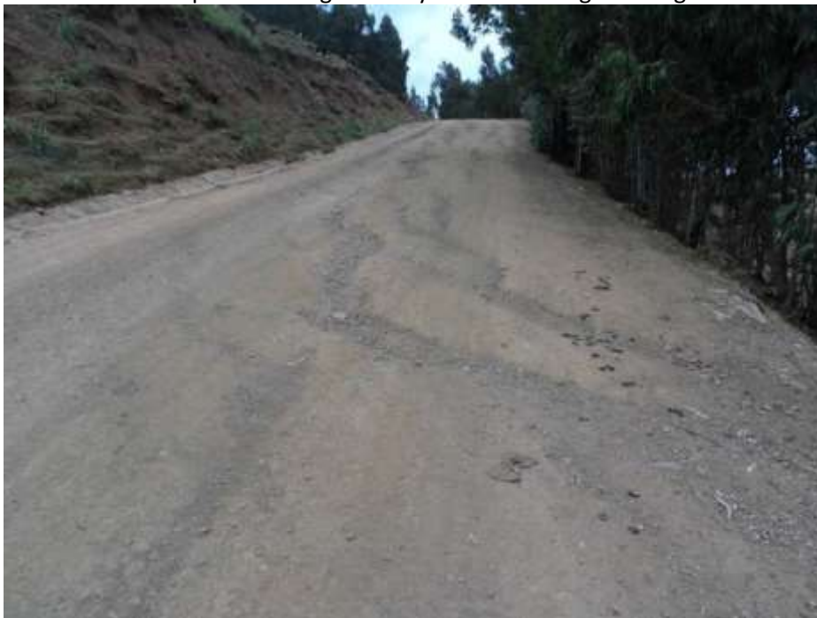
Figure A.9: Section of road with lined side-drain but showing excessive longitudinal (becoming transverse) erosion
