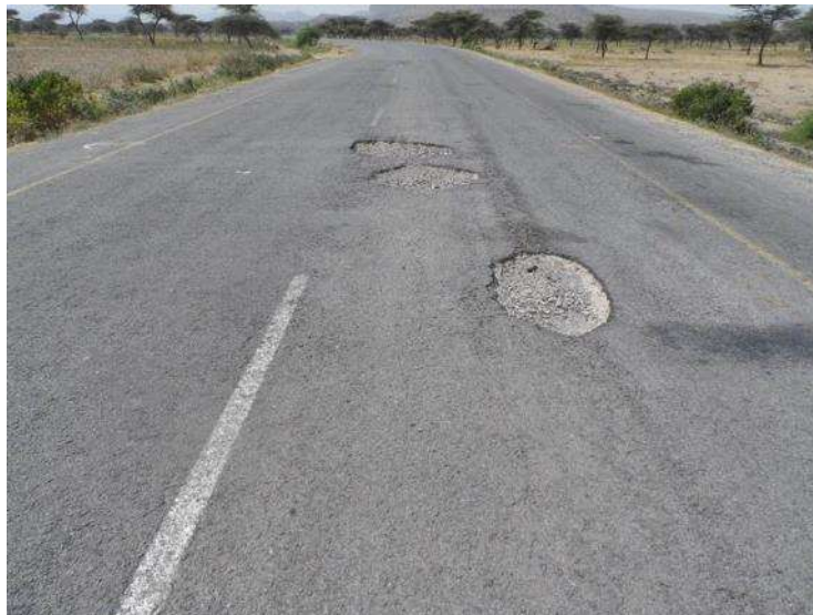
Figure A.23: Potholes on embankment over flood-plain
