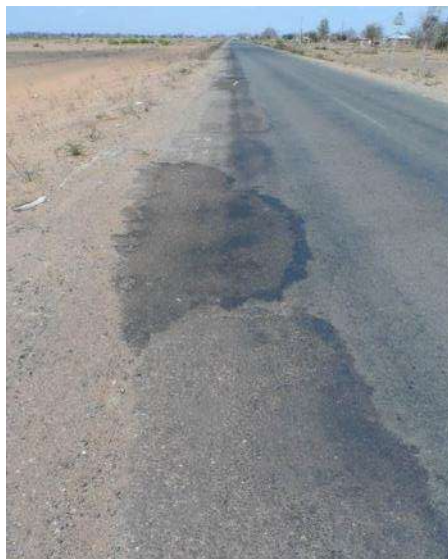
Figure B.22: Patches of outer wheel path failures in east-bound lane
