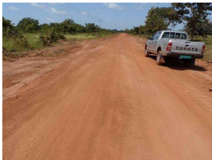
Figure C.2: Laterite wearing course with rudimentary drains – section still to be raised
