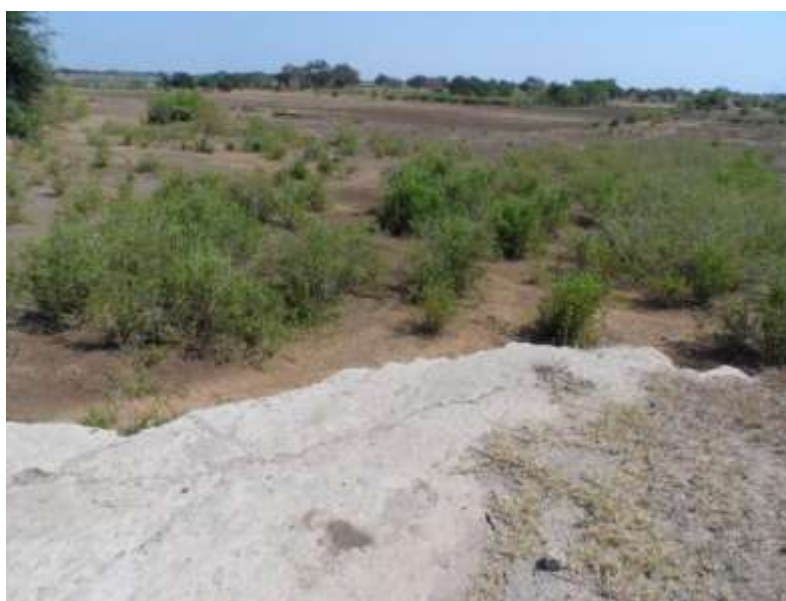
Figure B.11: Total loss of embankment due to flooding
