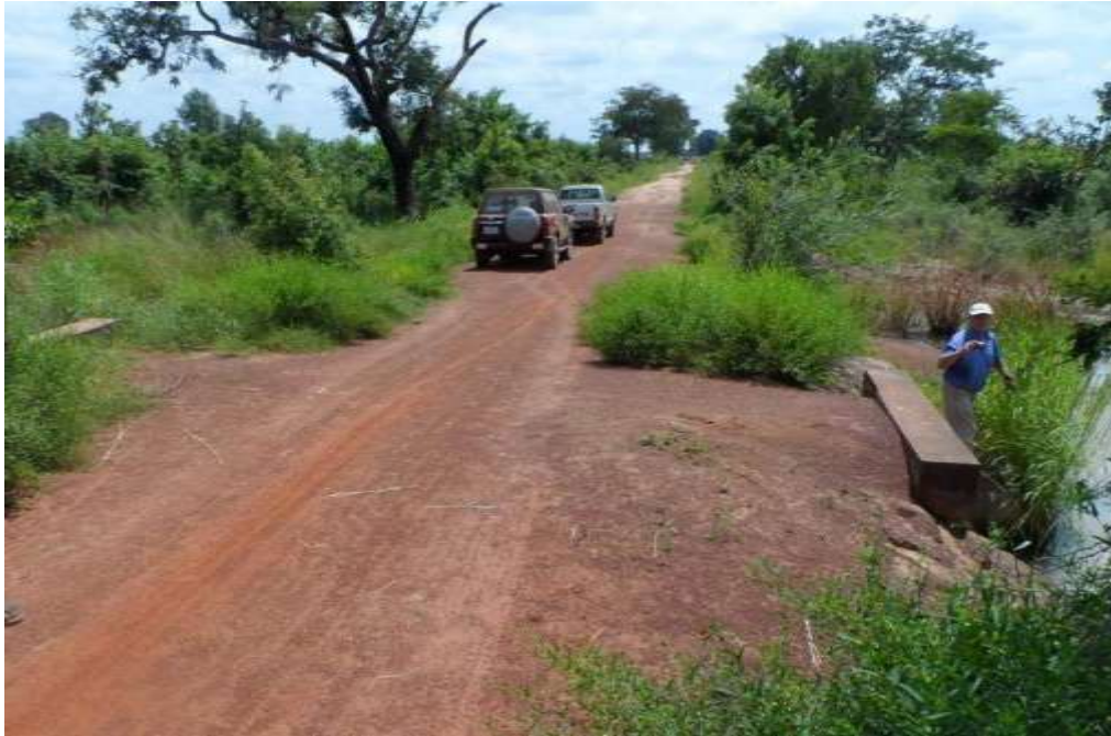
Figure 39: Erosion around culvert head-walls
