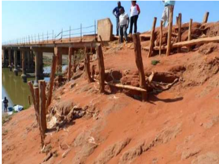
Figure B.10: Emergency repairs to approach fill on the Mobeira Bridge using sandbags and wooden stakes
