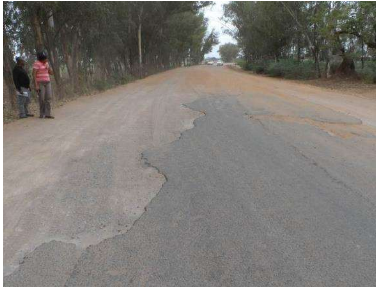
Figure B.21: Damage to and loss of surfacing caused by 2012 flooding
