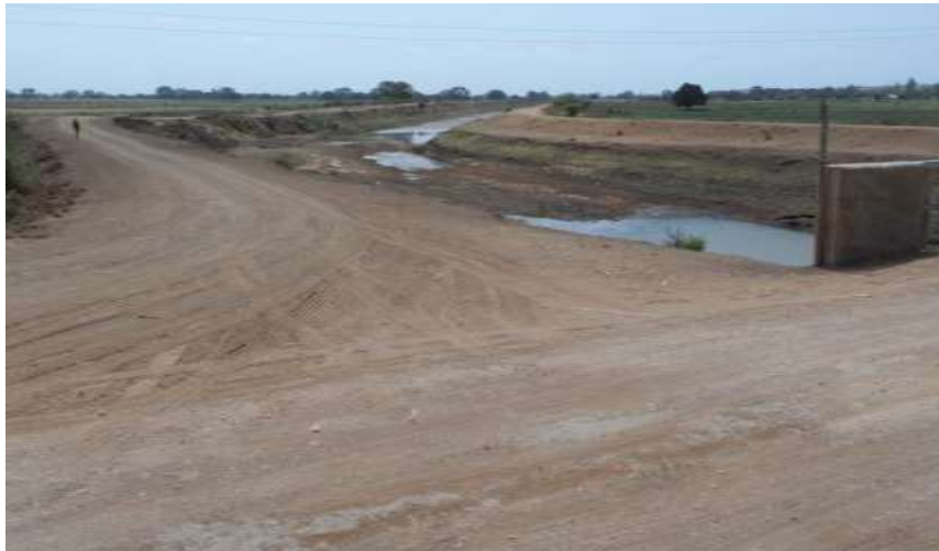
Figure B.41: Damaged road and fill caused by change in direction of river
