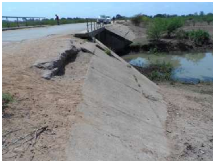
Figure B.24: Damage to small bridge approach fill, erosion protection and surfacing
