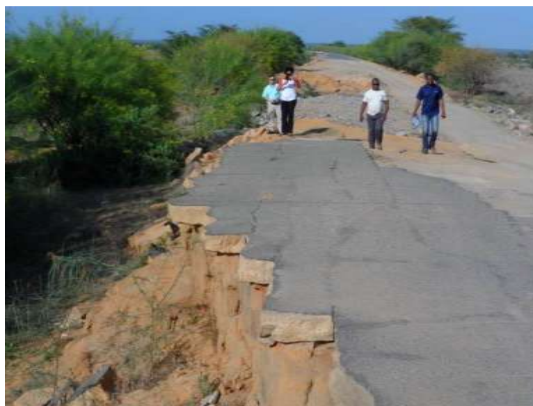
Figure B.3: Undercutting and collapse of pavement due to erosion of embankment during overtopping
