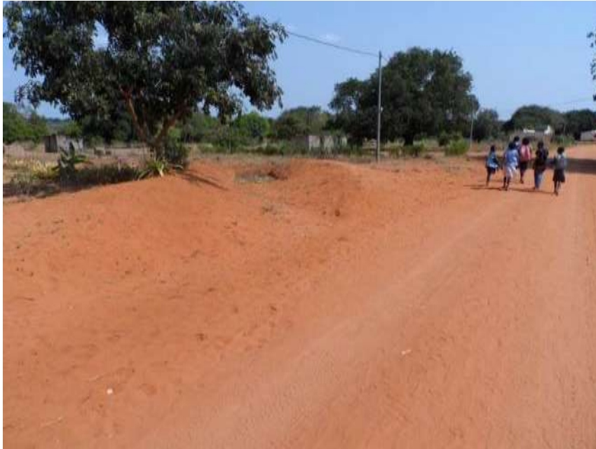
Figure B.37: Short mitre drain built up on both sides and at end during maintenance
