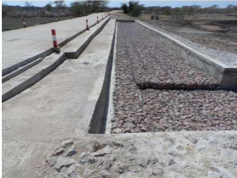
Figure B.15: Concrete drift with gabion lined stilling pond to minimise water velocities and erosion
