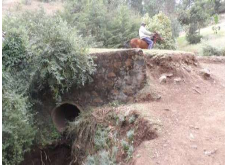
Figure A.12: Damage to head and wing-walls and pipe in culvert caused by adjacent erosion of the embankment
