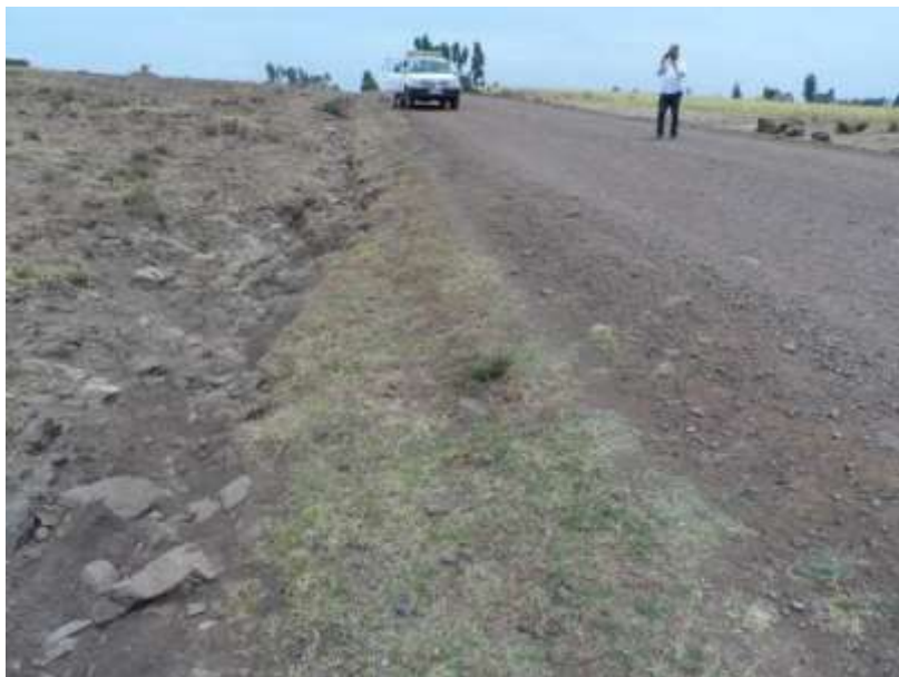
Figure A.5: Cinder gravelled road with erosion of side drains
