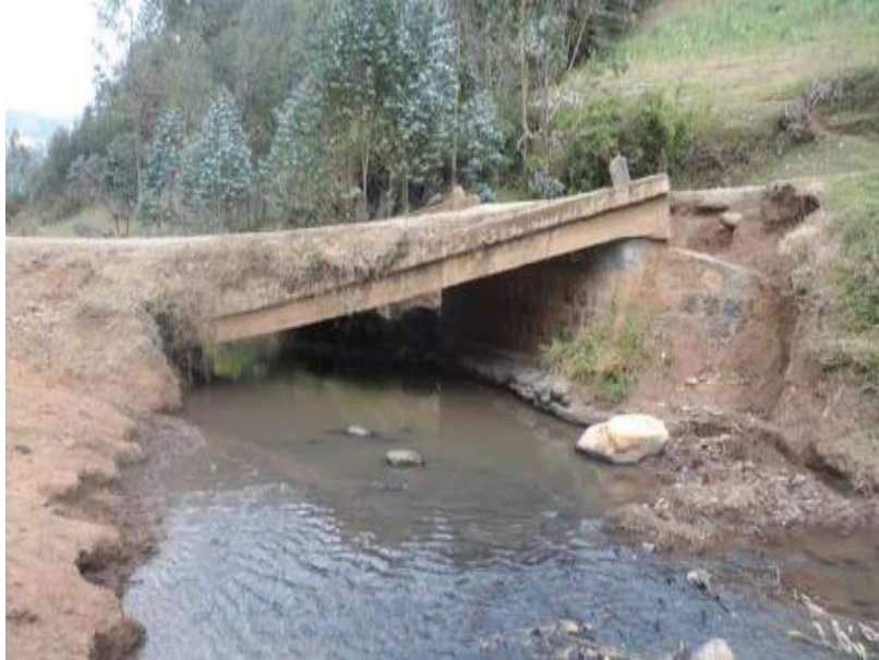
Figure 14: Collapse of small bridge and erosion of approach fill
