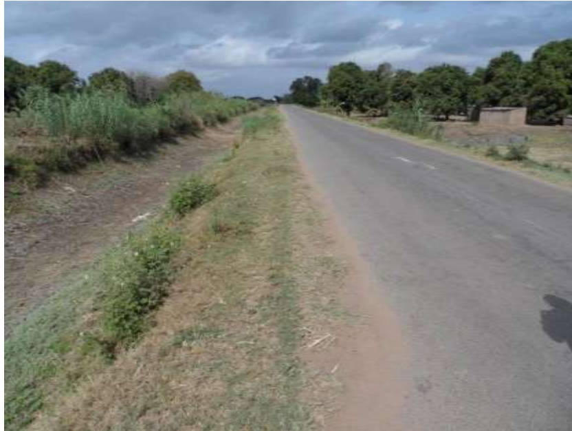
Figure B.18: Good section of Road R859 showing embankment and irrigation canal (empty)
