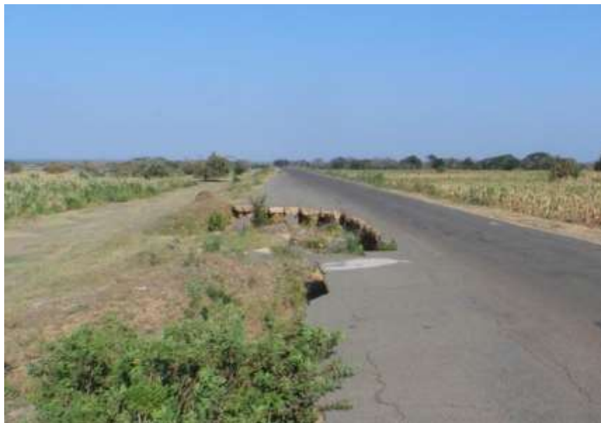
Figure B.7: Localised loss of road and embankment caused by turbulent flow around termite mounds
