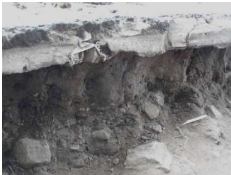
Figure B.19: Area of road showing Geocells and in situ material exposed by erosion of embankment next to road
