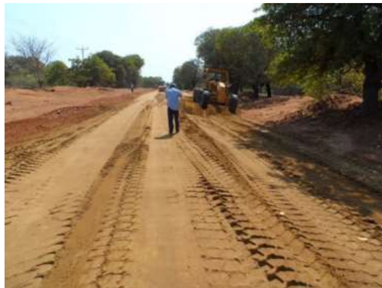
Figure B.29: Placement and compaction of subgrade material on Road R443 showing spoil piled at road edges
