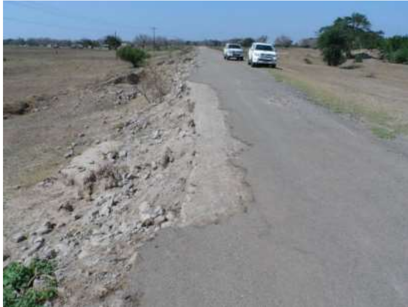
Figure B.12: Damage to embankment due to overtopping on approach to site in photograph above
