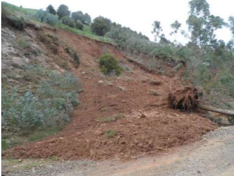
Figure A.10: Landslide at km 44.6
