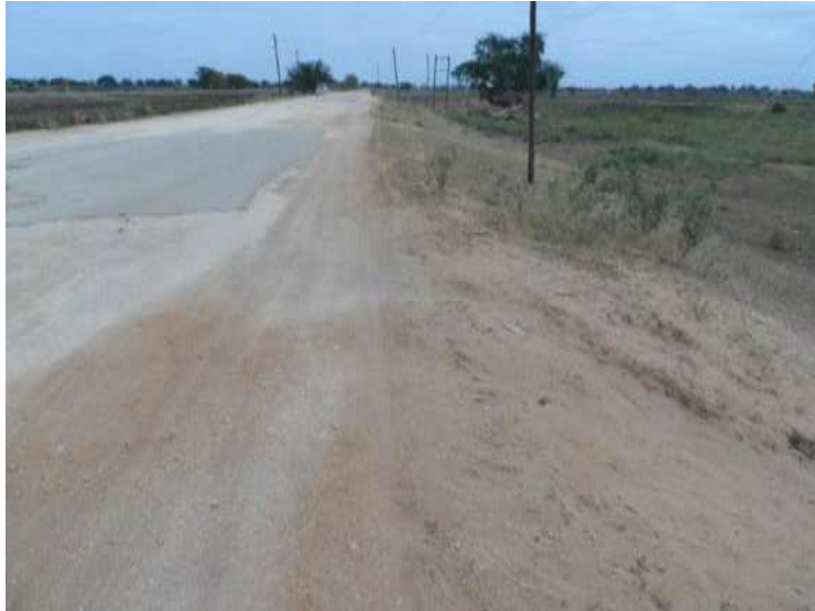
Figure B.25: Loss of seal and damage to embankment
