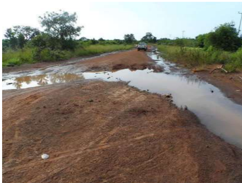
Figure C.17: Poor drainage due to perched water tables and ineffective pipe culverts
