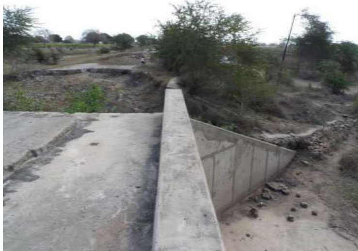
Figure B.17: Loss of approach fills on three consecutive bridges
