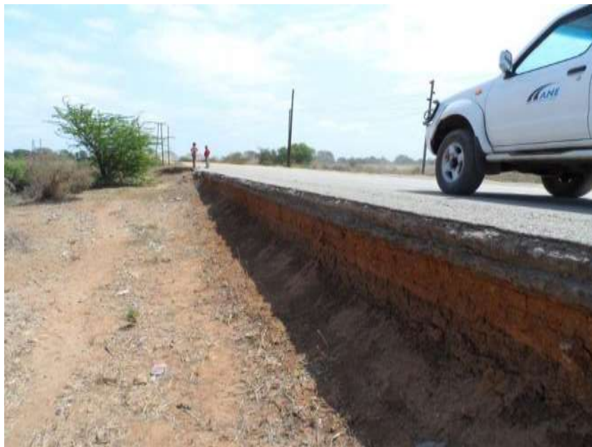
Figure B.36: Undercutting of downstream part of road due to water flowing across it
