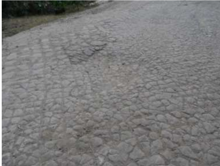
Figure B.20: Area of Geocells with total loss of seal and development of pothole in central part of photograph
