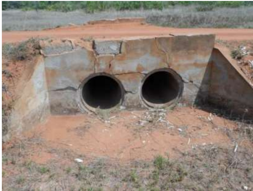
Figure B.39: Culvert allowing equalisation of water where road has severed floodplain area – note damage and potential for further damage when soaked
