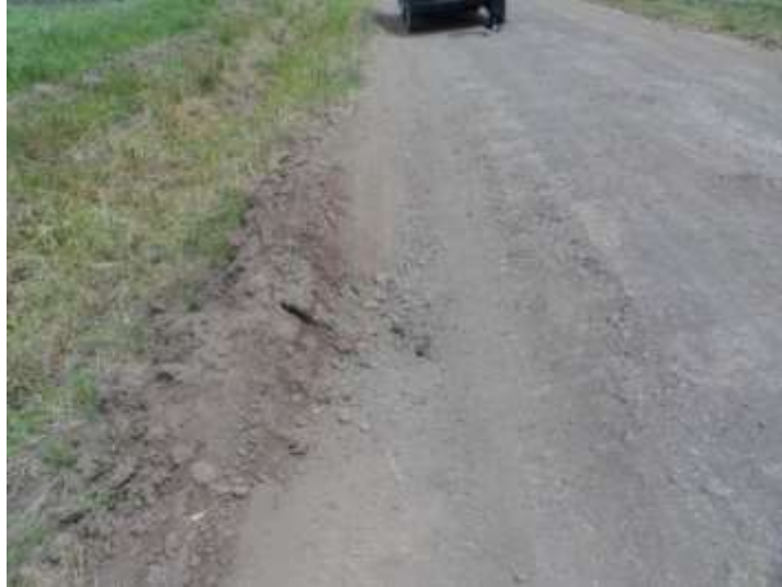
Figure A.6: Shear failure of subgrade at point of water accumulation
