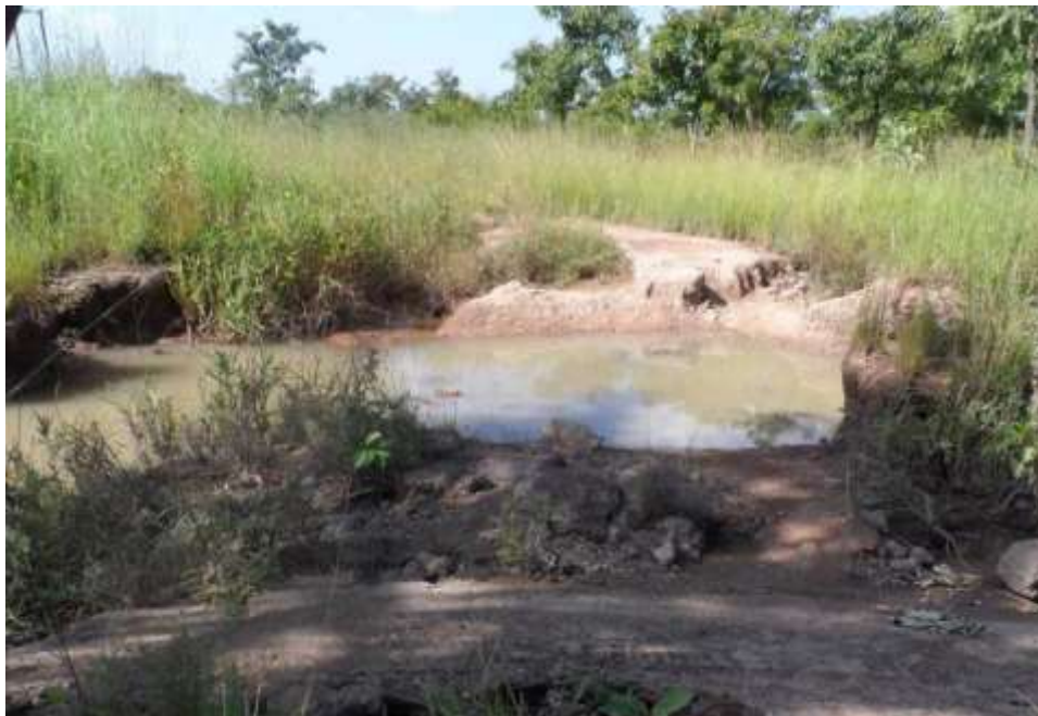
Figure C.4: Site of culvert washed away and due to be replaced
