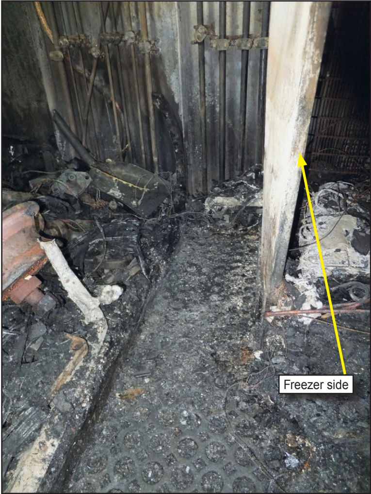
Figure 5: Location of source of fire
