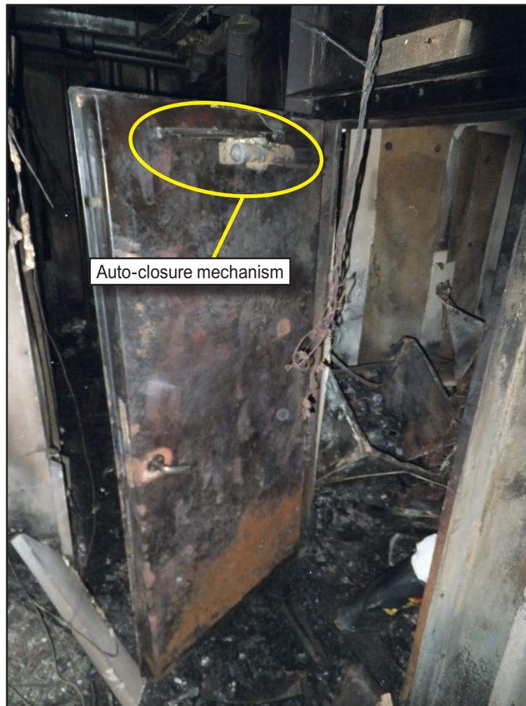
Figure 3: Galley fire door with auto-closure disconnected
