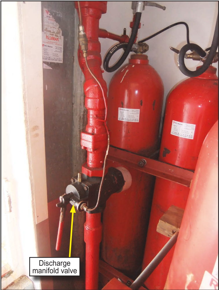
Figure 7b: CO 2 manifold valve
