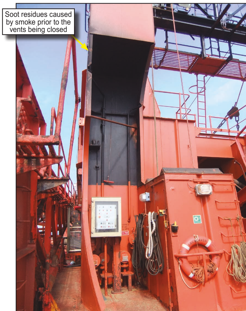
Figure 2: Port engine room vent
