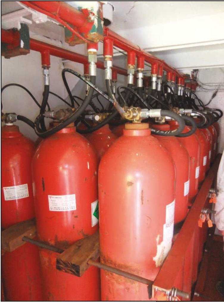
Figure 5: CO 2 cylinder room
