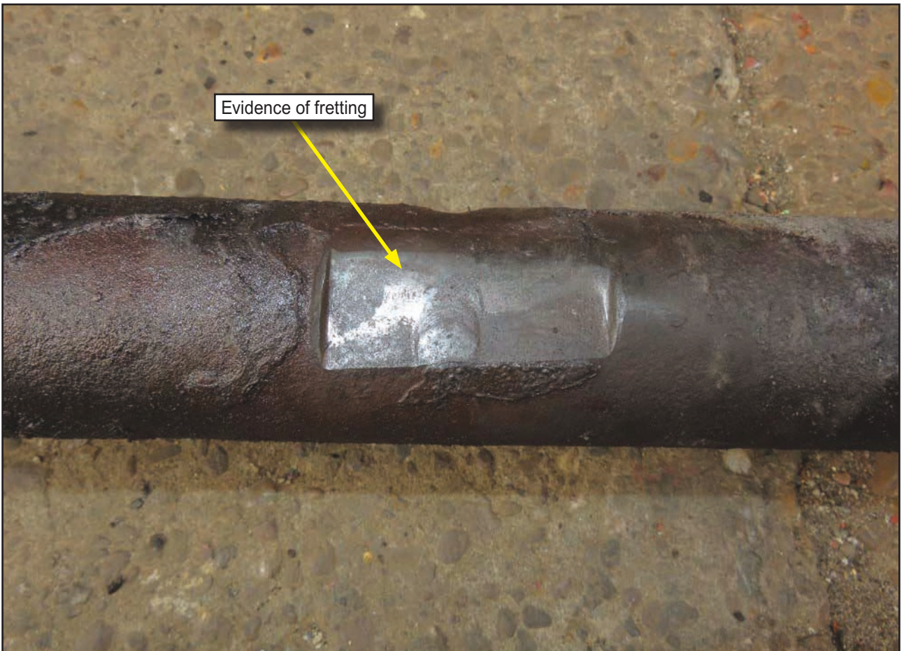
Figure 12b: Evidence of pipe interference
