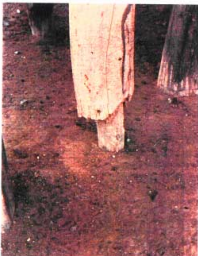
Plate xviii. Termite damage to the sapwood of mopane posts; note the resistance of the heartwood (see page 21)
