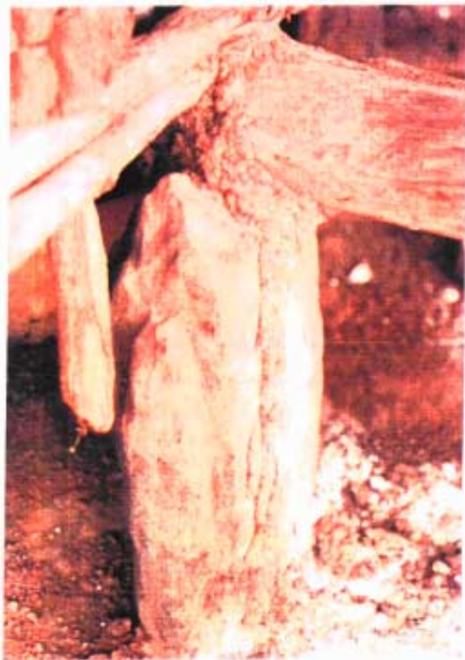
Plate ix. Rock support in a grain store showing termite track up the rock and on the surface of the horizontal timber bearer (see page 15)
