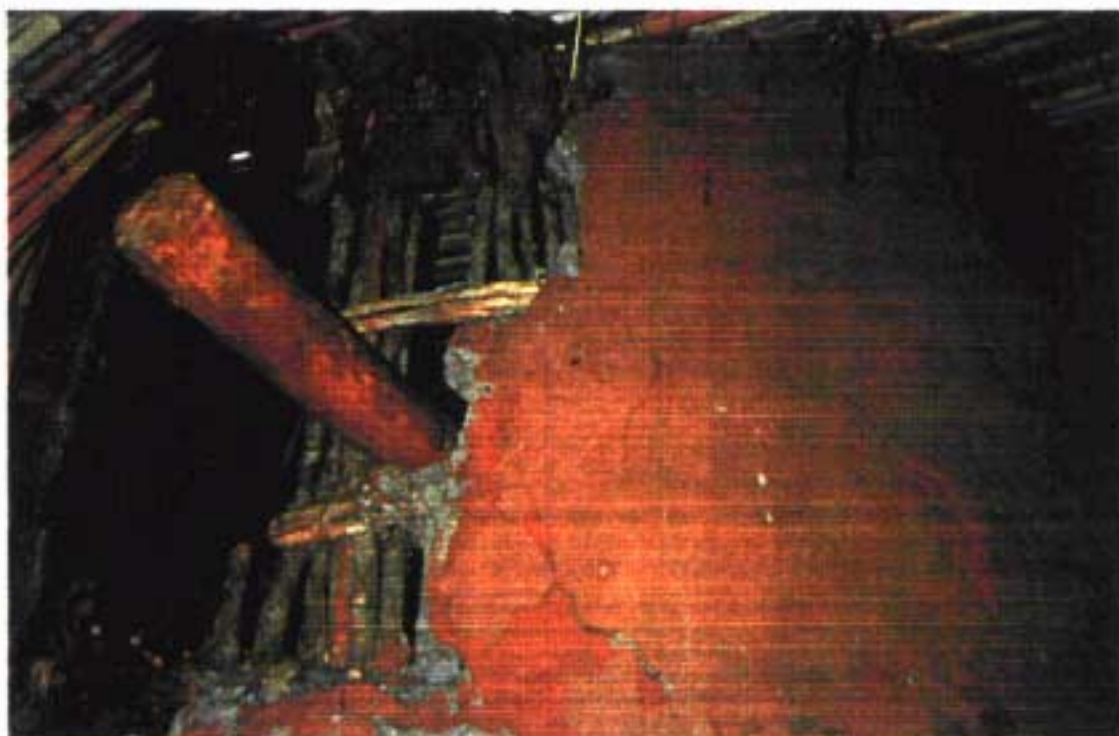
Plate xxv. Poorly maintained store; note the failed external plastering (see page 35)
