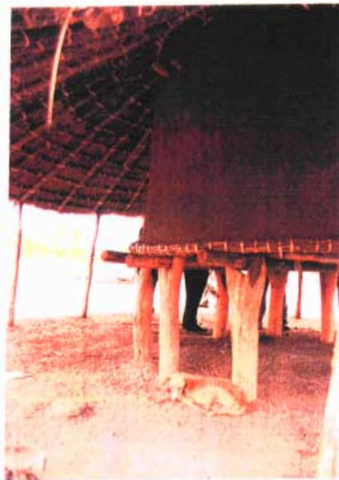
Plate x. Mopane main posts showing the use of forked trunks to support the main horizontal floor bearers (see page 16)
