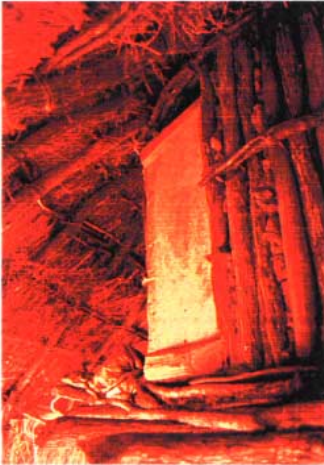
Plate xxiii. Ill fitting store door allowing access for infestation and vermin (see page 34)
