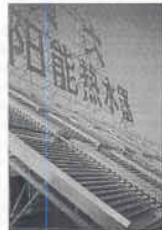
Solar Hot Water Installation, Near Hangzhou, China
