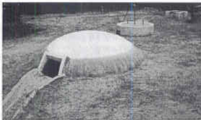
School Biogas Installation, Zimbabwe
