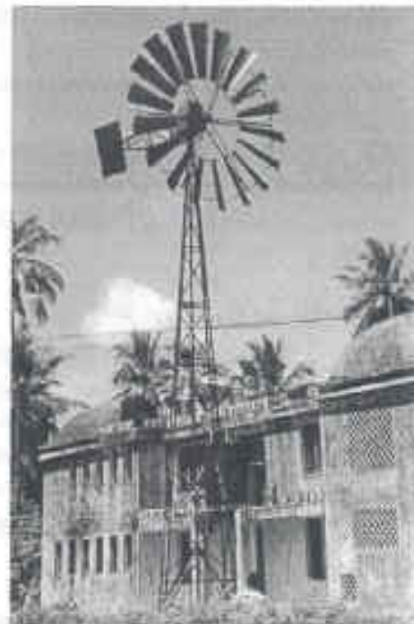
Wind Powered Water Pumping, Kenya
