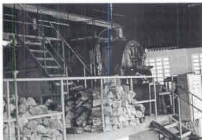
Biomass (wood) boilers, Tea Estate, Kericho, Kenya
