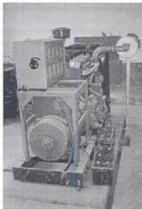
Spark Engine for Converting Biogas to Electricity
