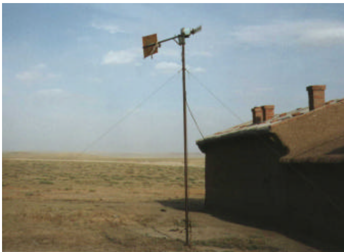
Wind generator located to rear of house
