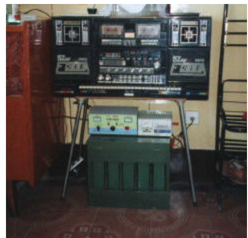
Inverter, controller and batteries
