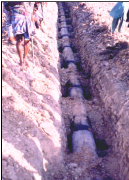
Buried pipe system
