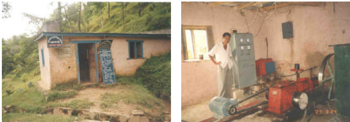
Figure 5. Micro-hydro powerhouse at Pinthali
