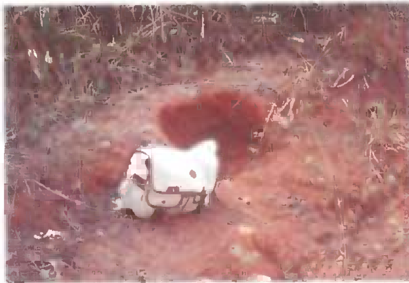
Figure 21. A small borrow pit (?), used to repair small road gullies, Lome village
