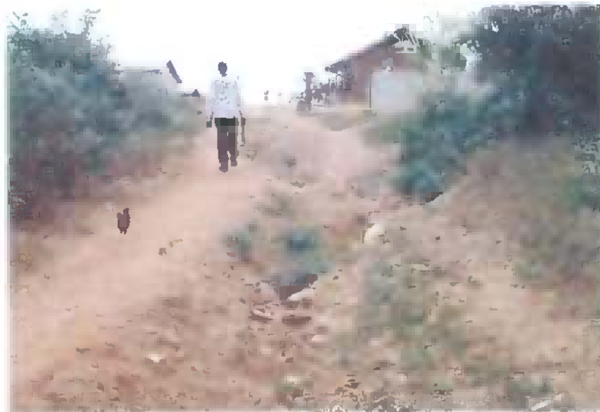
Figure 25. Gully at the start of path 1, Awurabo village. Some gully control may have been undertaken with rock placement.
