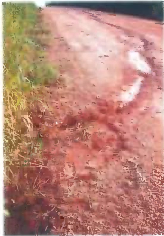
Figure 6. Road gully developed on the slope on the far slope in Figure 5, Adabra village
