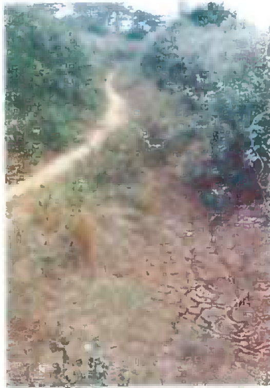
Figure 26. A section of Path 1 (Awurabo village) widened by a tracked vehicle, showing signs of swelling clays (i.e., instability) and gulying
