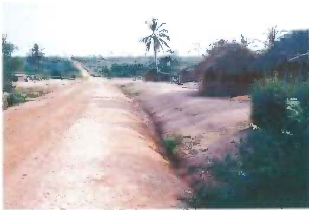
Figure 5. Road-side drain over-deepening due to surficial erosion, Adabra village looking South.
