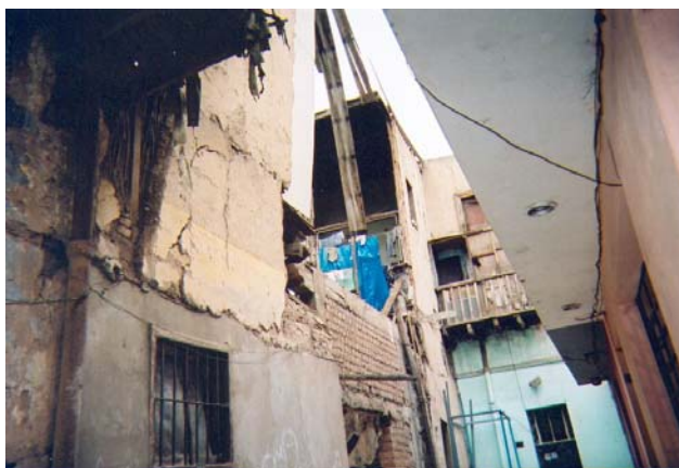
Photograph 3. Dilapidated Tugurio in Lima, Peru
