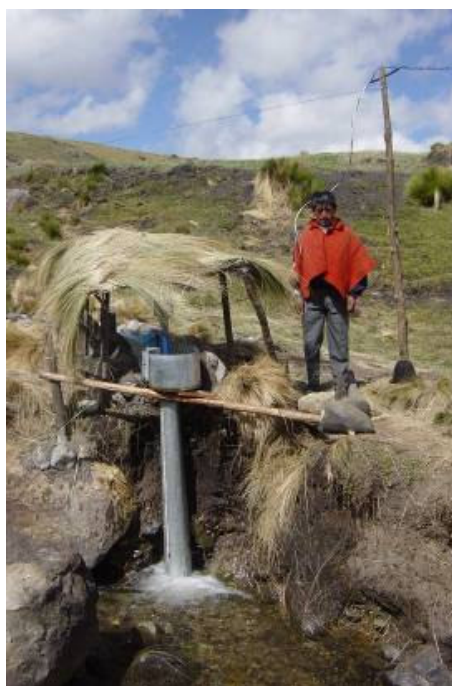
Figure1 – Pico-hydro installed in Ecuador for family use
