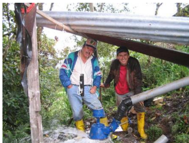
Figure 5 – Vietnamese 200 W medium-head pico-hydro 'turgo' unit installed in Ecuador
