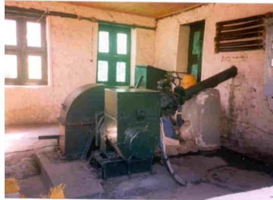
Interior of Ghandruk powerhouse
