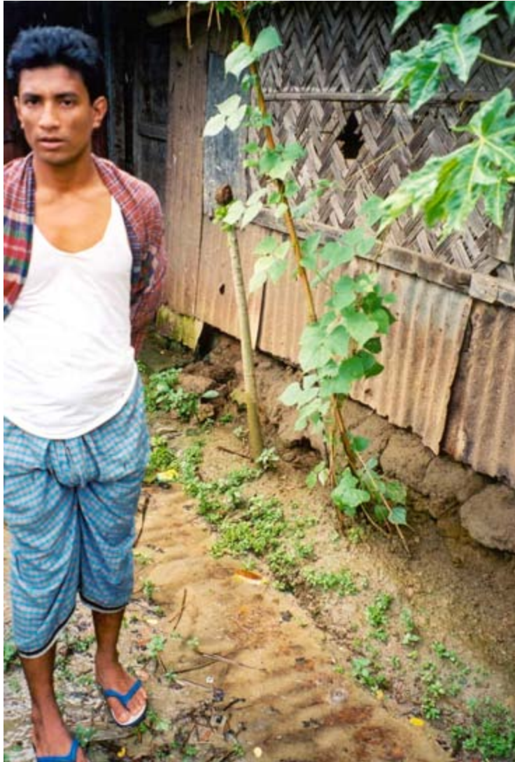
Figure 10. Photograph of rodent burrows in house foundation
