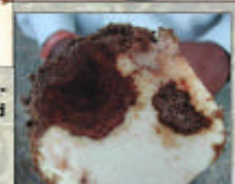
Dry-rot with insect damage
