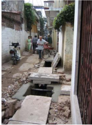
Figure 6 Upgrading of sewerage in Quynh alley, Quynh Loi ward, Hai Ba Trung district
