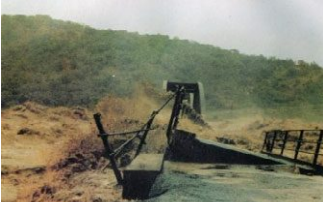
Flood damaged bridge in South Africa.
