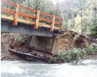
Flood damaged bridge in the USA.
