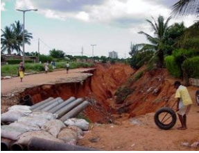
Flood damaged road in Mozambique.
