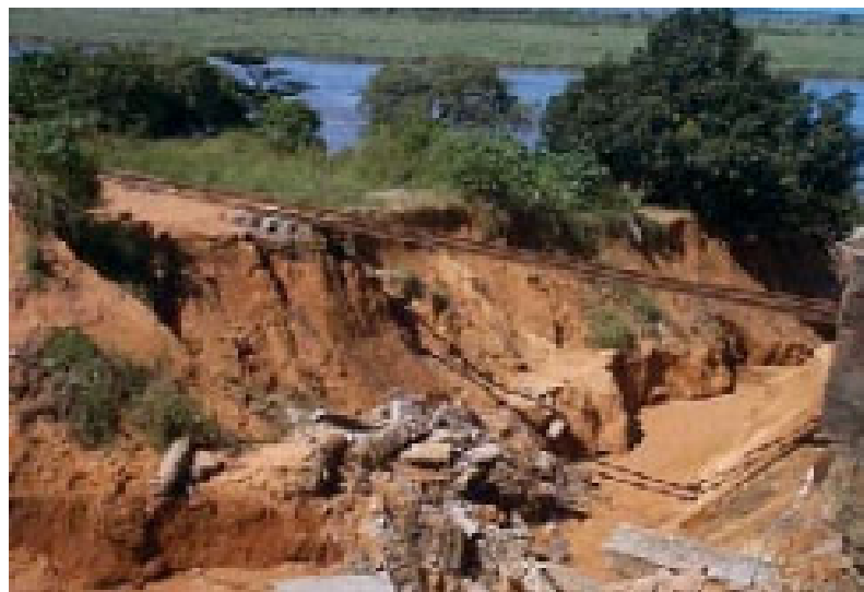
Figure 6.1 Damaged railway line embankment in Mozambique
