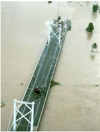
Bridge at Xai Xai in Mozambique during the 2000 floods.
