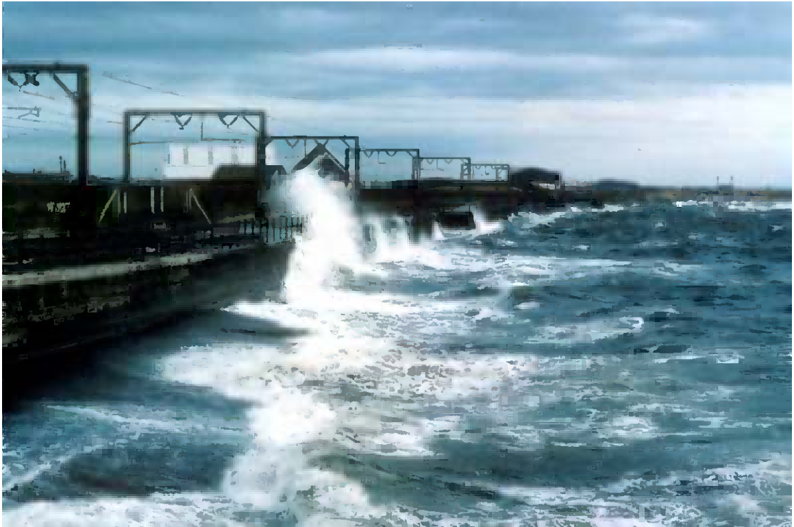
Figure 1.7 Overtopping of sea walls in the UK
