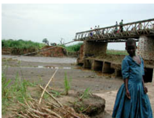
Flood damaged bridge in South Africa.
