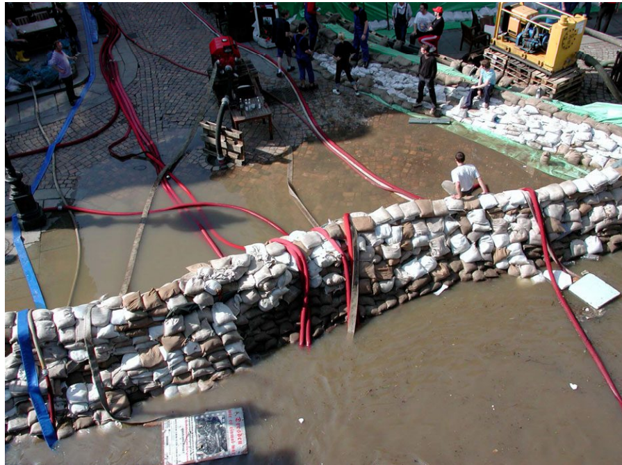
Figure 5.4 Use of sandbags in Dresden, Germany during the 2002 floods
