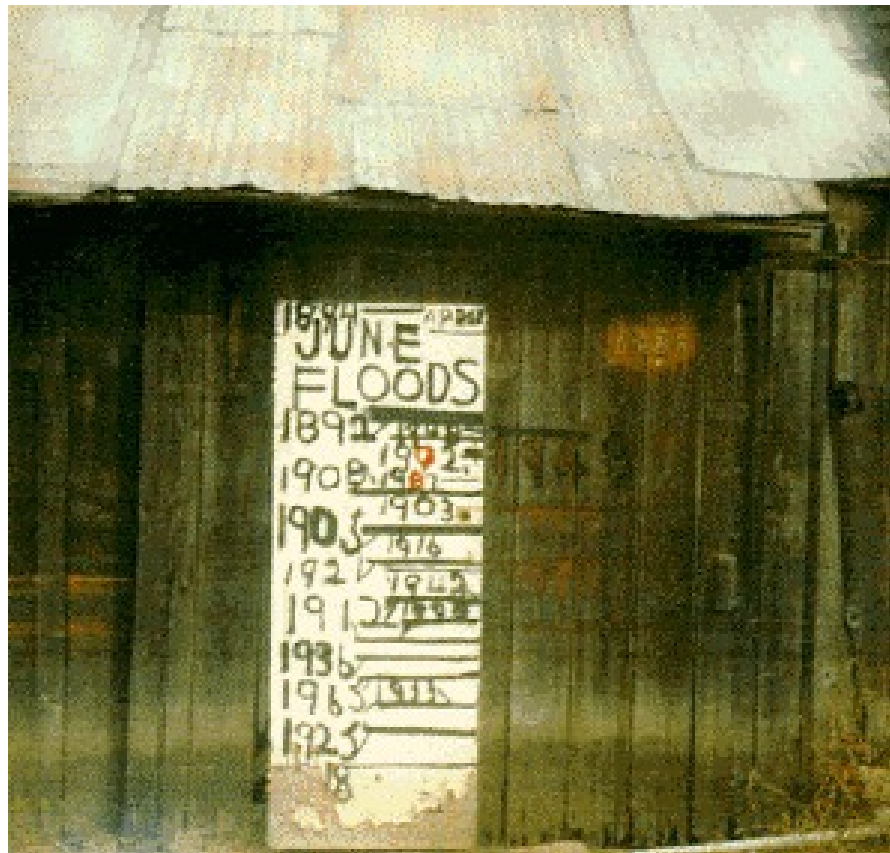
Figure 2.13 Flood marks on a building in Canada
