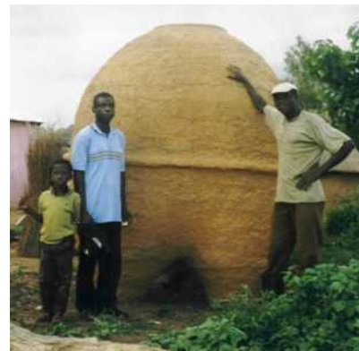
Figure 15 Elephant size legs of Saboba/Chereponi mud silos set on flat, firm and well balanced stones
