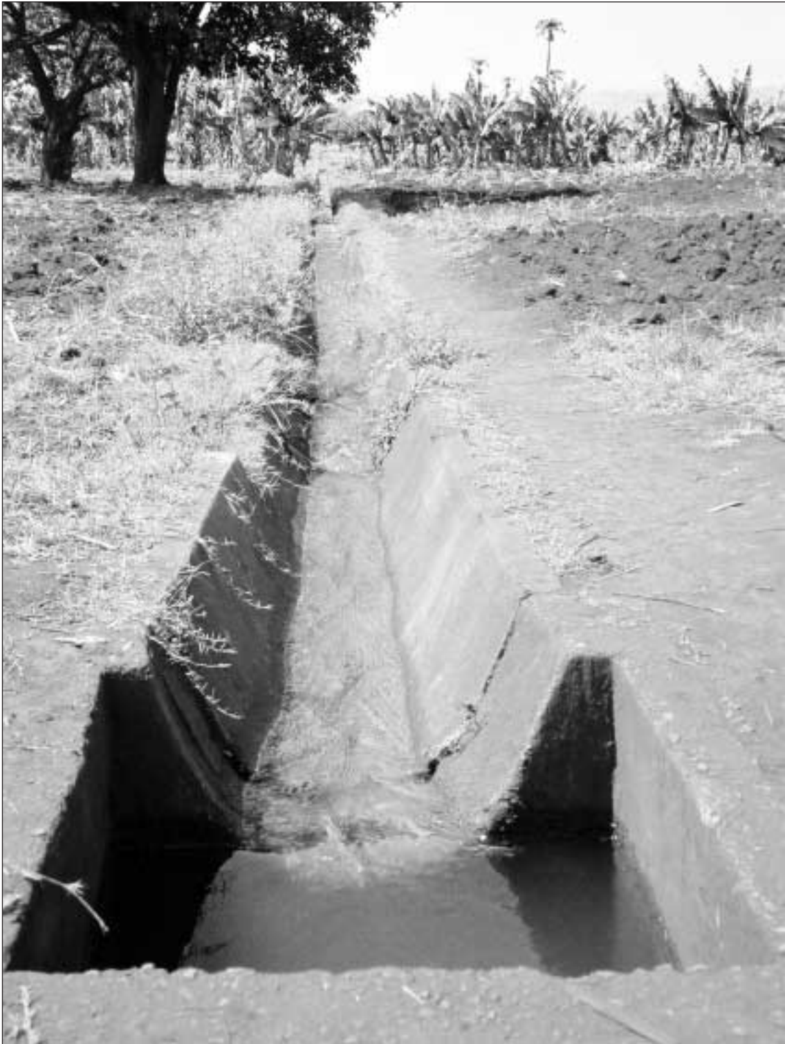
Sub-canal at the Khumbe irrigation scheme in South Africa. © Rob Hope
