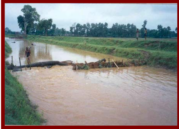
Improper diversion of water by creating obstruction against flow
