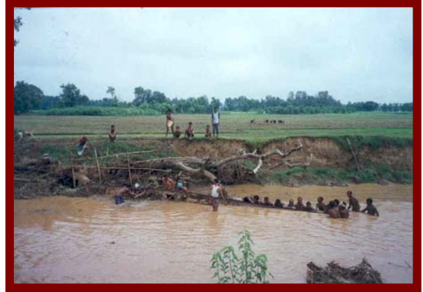
Creation of obstruction in progress for improper diversion of water against flow
