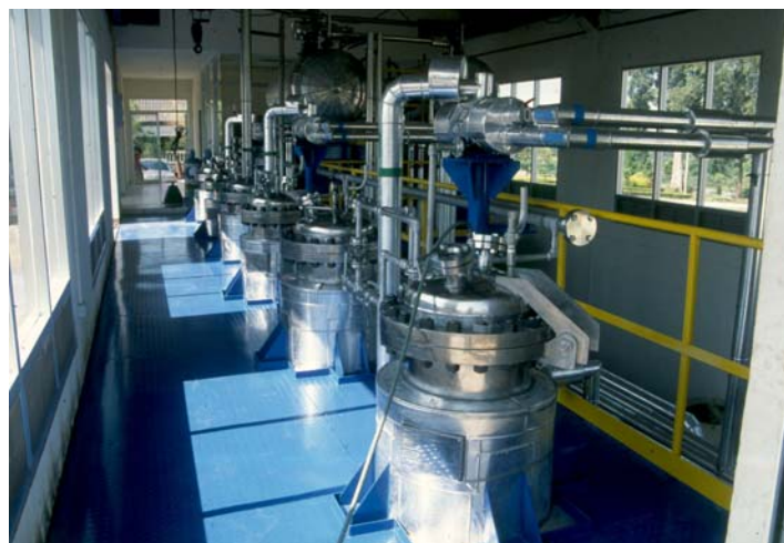
Commercial HFC-134a based extraction facility, Phurua Natural Oils Ltd, Thailand. (Courtesy of Peter Wilde Associates Ltd).
