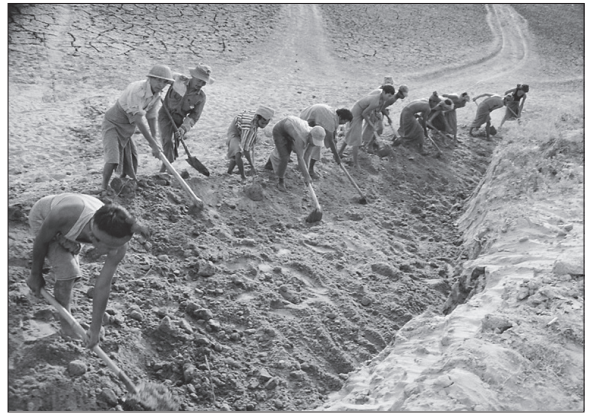
Workers repair soil by traditional methods to protect from soil erosion and dry land Myint Thar Zi, Myanmar.
