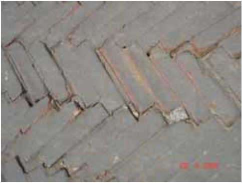
Missing Sand Infill to Joints
