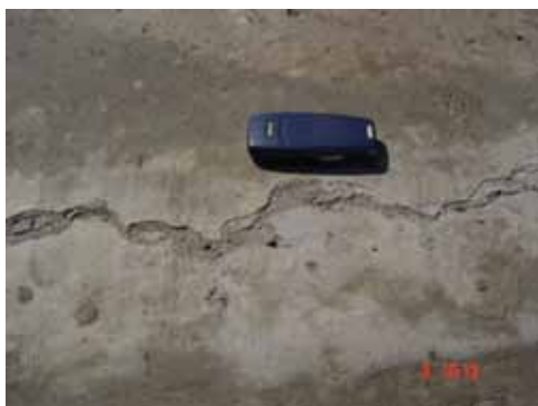
Cracked Concrete Pavement
