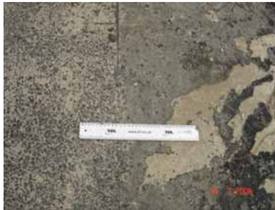
Bituminous Pavement Bleeding
