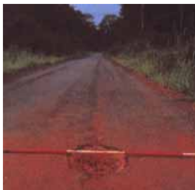
Pothole in a Bituminous Chip Seal
