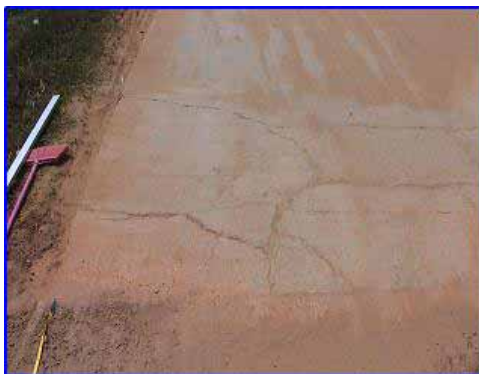
Severely Damaged Concrete Pavement
