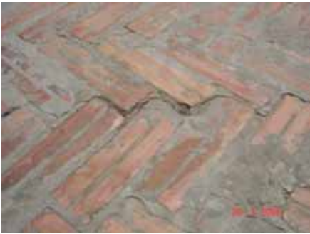
Cracks in Brick Joints
