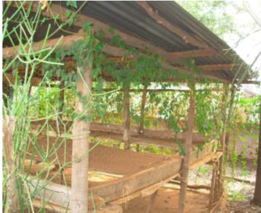
Figure A10.1 Two views of an abandoned collection shed owned by the first group of small-scale growers in Kenya to be EurepGAP certified under option 2.
