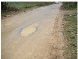
Potholes on the bitumen road surface
