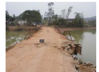
Abutment Defects cause slipping on road
