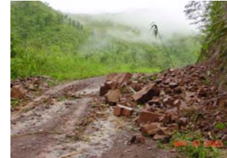
Slipping on cut slope
