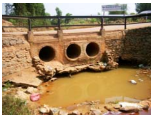
Erosion on apron
