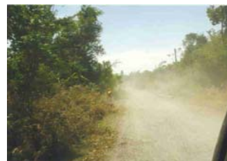
Dusty on the gravel road surface as vehicles cross
