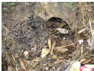
Culvert is blocked by debris
