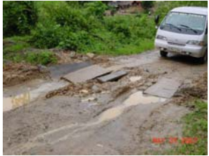
Soft Spot because of culvert defects
