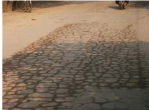
Crocodile crack on the bitumen road surface
