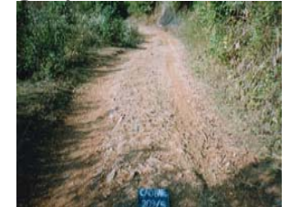
Vegetation growth excessive on road shoulders and side drain is silted
