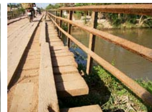
Planks on the wooden bridge disappeared
