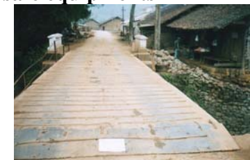
Bridge without railing, without signal board
