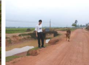
Erosion on fill slope
