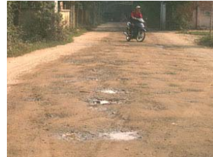
Potholes on the Macadam road surface
