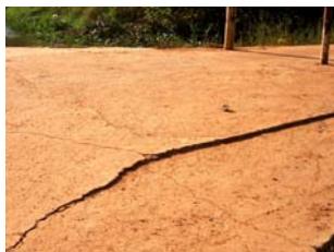
Crack concrete slabs on the road
