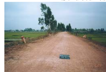
Stake disappeared, broken
