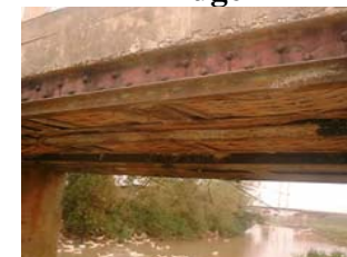
Steel Beam is rusty
