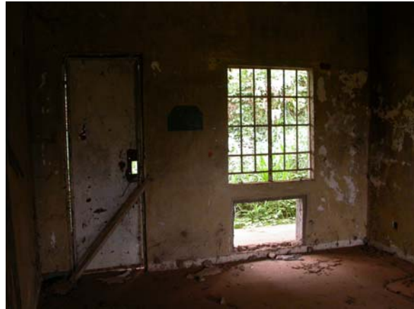
The MAFFS offices in Makeni were taken over by the Revolutionary United Front (RUF) rebels during the war. Everything was stolen, including the aircon units .
