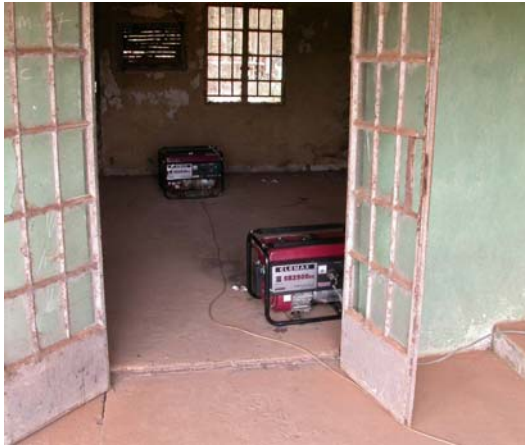
Twin generators, hired from town, that powered our training course in an adjacent room
