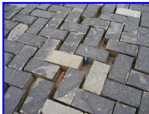
Plate 4: Seal Eroded from Concrete Block Paving: Sand Joints
