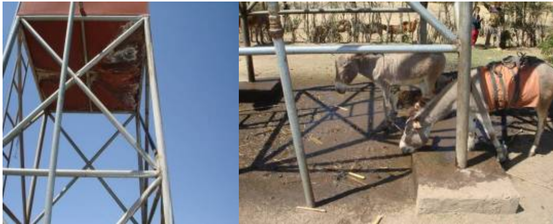
Figure 4.7: Cattle drinking water below the severely leaking tanker
