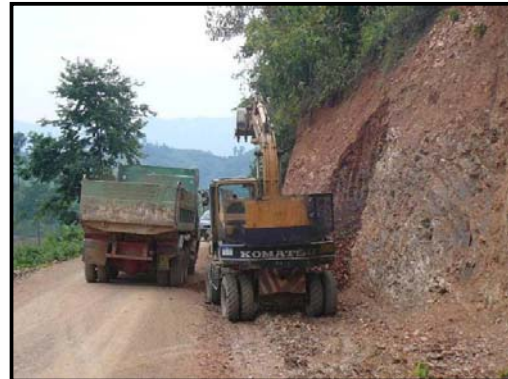
Plate 4 Over-steepening of cut-slopes in order to obtain out-of specification gravel using heavy trucks.
