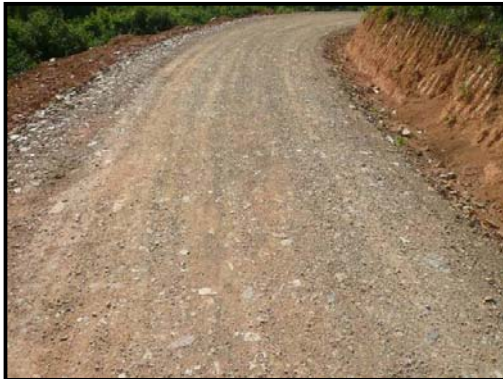
Plate 3 Coarse out-of specification wearing course materials evident in this section
