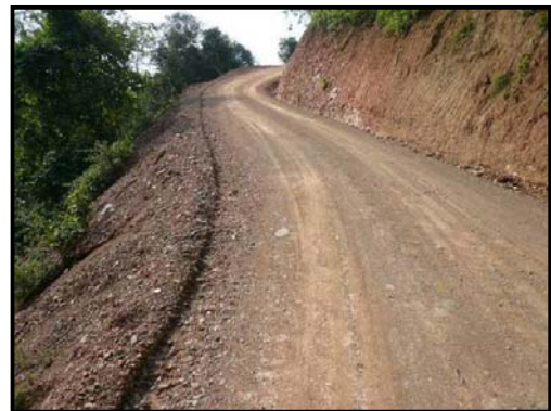
Plate 6 Poor compaction in shoulders evidenced by ruts and tyre marks
