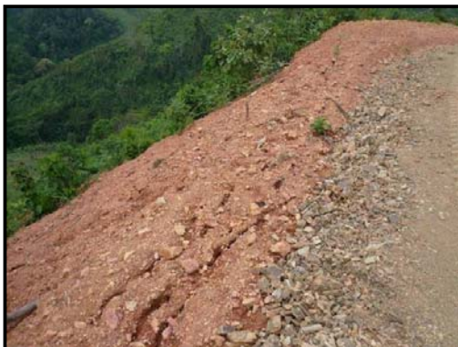
Plate 5 Tension cracks evident in failing materials dumped below road
