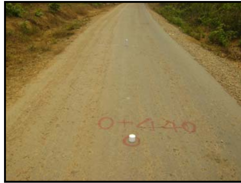
Figure 4.1 Defects in Otta Seal – possibly construction related
