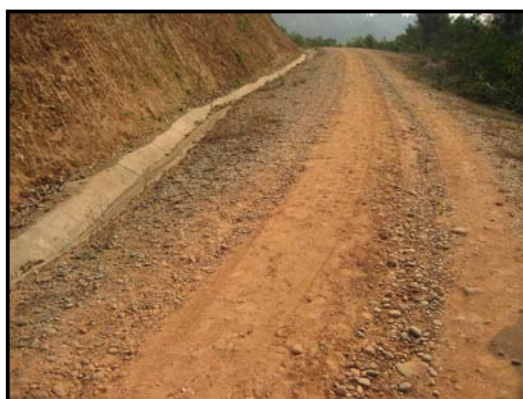
Figure 5.3 Eroded gravel on steep section of NEC package II road 201. Shape prevents run-off into well constructed drain
