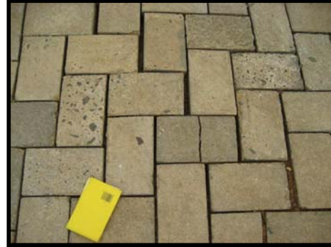
Figure 4.6 Eroded badly spaced joints. One cracked block
