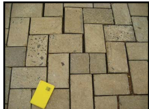
Figure 10, Eroded badly spaced joints with one cracked block
