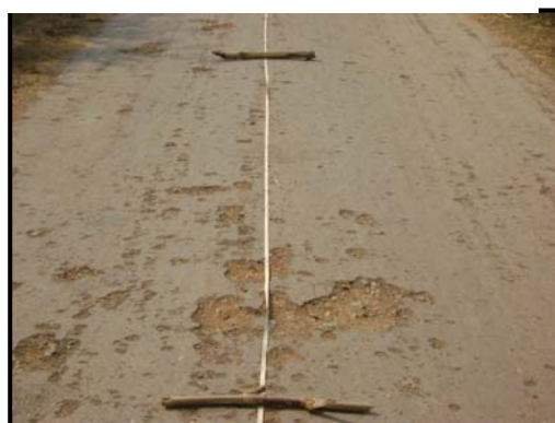
Figure 4, Seal erosion and shallow potholes - Road 1032.01
