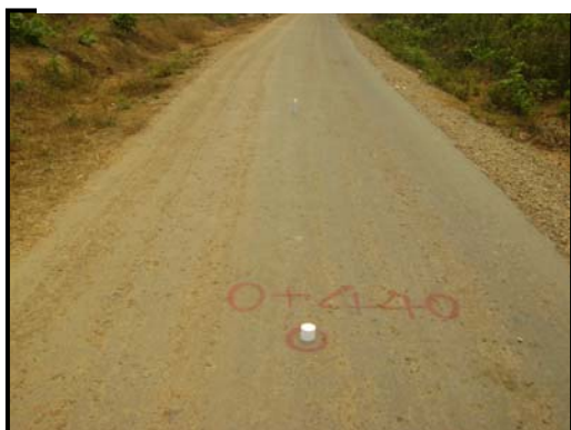
Figure 3, Defects in Otta Seal – possibly construction related.
