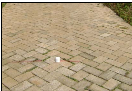
Figure 9, Grass growing within joints may loosen blocks.
