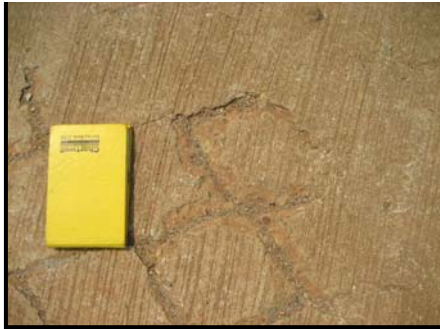
Figure 7, Erosion adjacent to cell boundaries.
