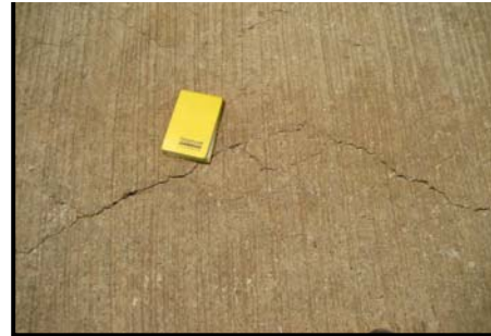
Figure 8, Cracks in surface screed following cell boundaries.
