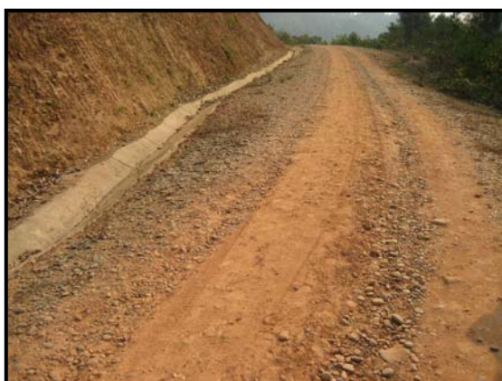
Figure 15, Eroded gravel on steep section of NEC package II road 201. Shape prevents run-off into well constructed drain.
