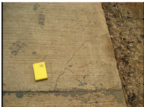
Figure 11. Typical corner edge crack in concrete slab.
