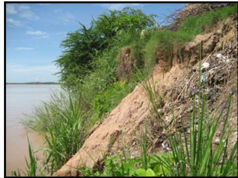
Figure 4.3 River Bank Erosion
