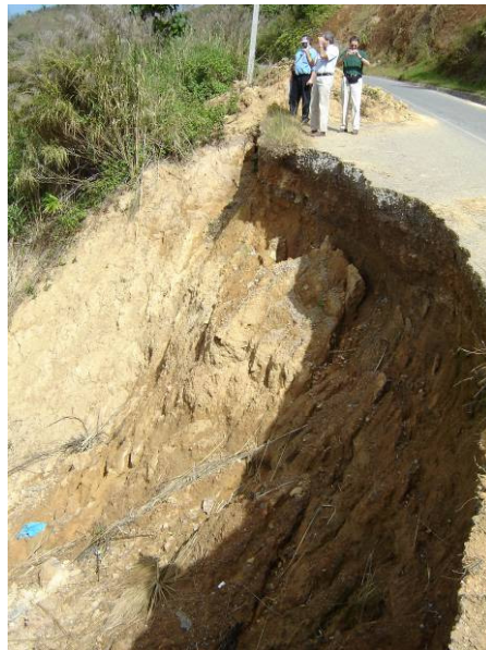
Typical below-road landslide
