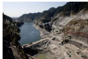
Lower Subansiri dam and power station in Arunachal Pradesh, Northeast India/ Tania Ghosh - Panos London
