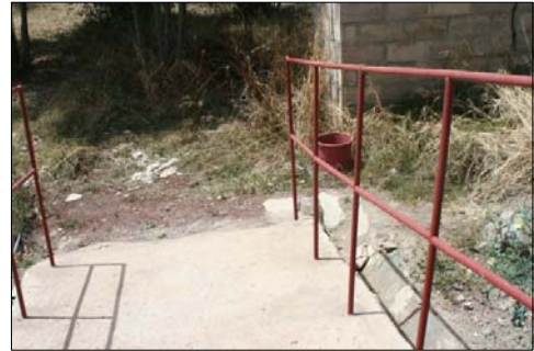
Figure 4 This latrine has guide rails but the approach is inaccessible
