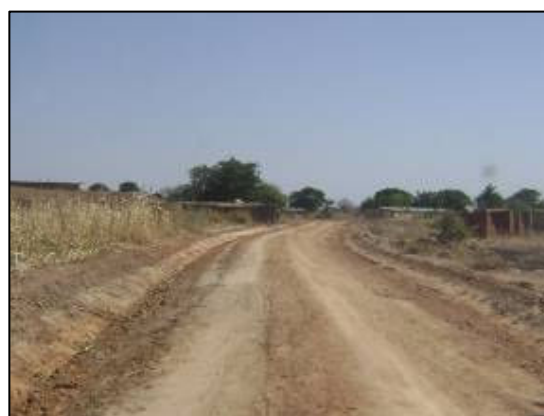
Section of Mtita – Nchinila road that has been heavily graded
