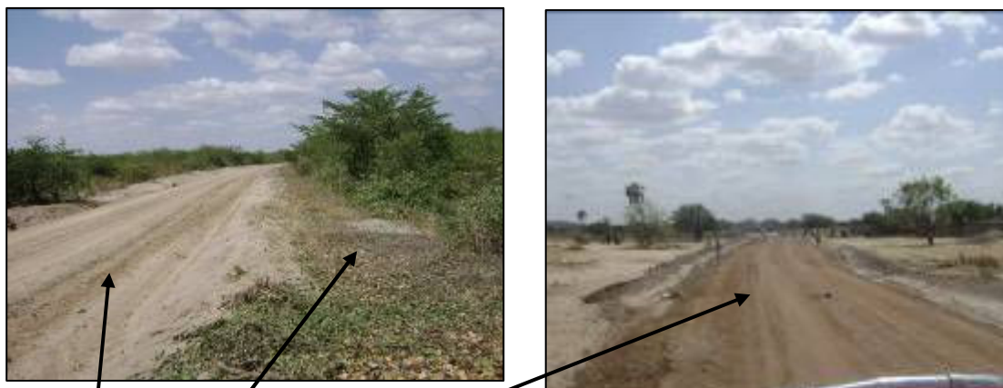
Light grading, bush clearing and spot gravelling being done on Bahi Sokoni – Chimendele road
