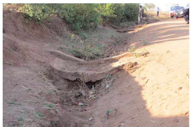
Section of road on relatively steep gradient showing severe erosion of drain downstream of scour check
