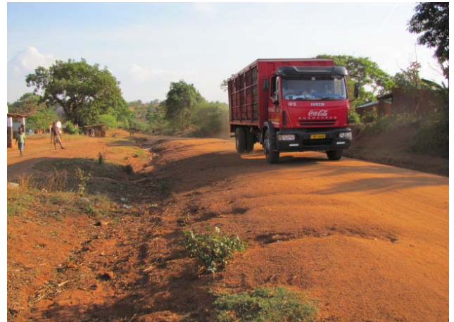
Section of gravel road on moderate gradient showing some rutting, deformation and drain erosion
