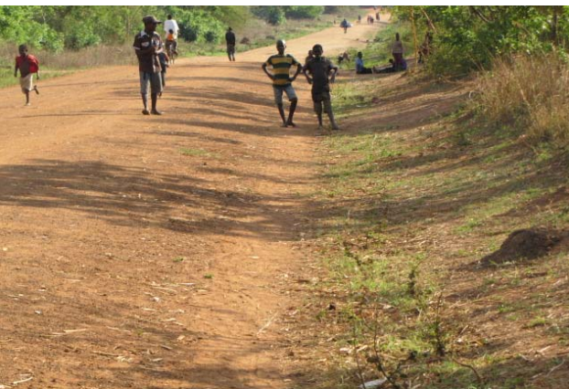
Well formed and drained, gravelled section of road exhibiting gravel loss after one year
