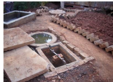
Figure 5. Fixed dome digester at Nsambya Babies Home in Kampala
