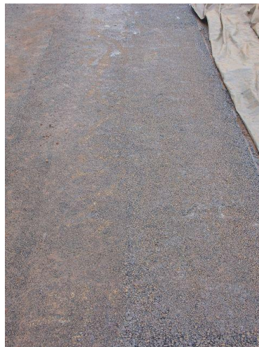
Good joint, hardly visible
