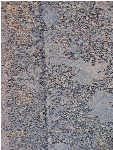
Joint too open, requires emulsion and crusher dust to seal
