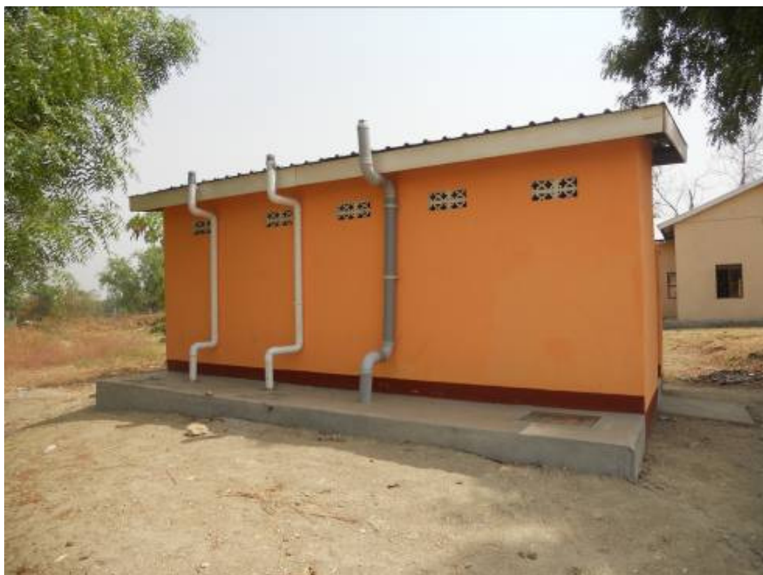
Plate 1 VIP latrines and washrooms show cranked vent pipes
