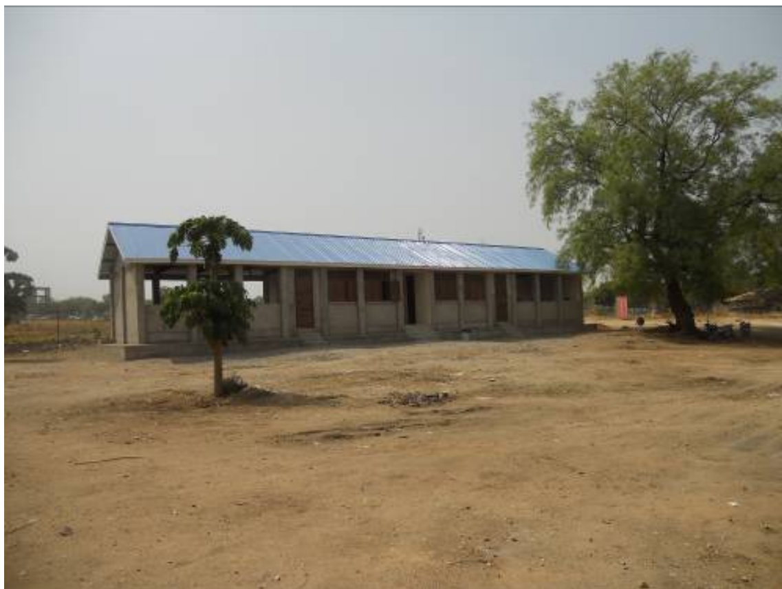
Plate 4 YEP Centre showing poor location and lack of access veranda
