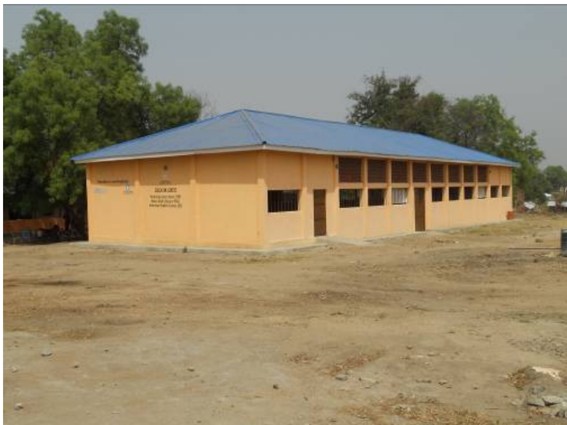
Plate 7 Central hall showing lack of protection to openings in walls
