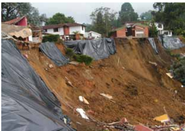
Figure 2: Slope Failure Source: Gonzalo Duque
