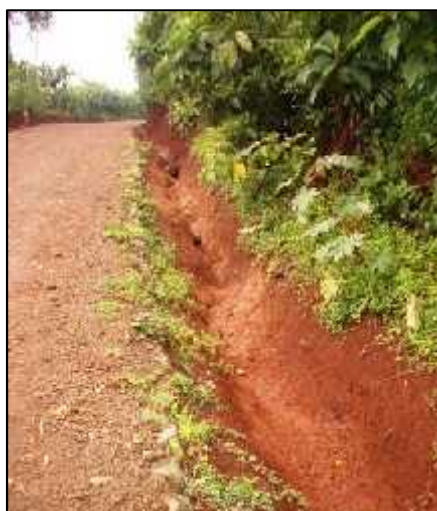
Eroding side ditch on URRAP road with no check dams.
