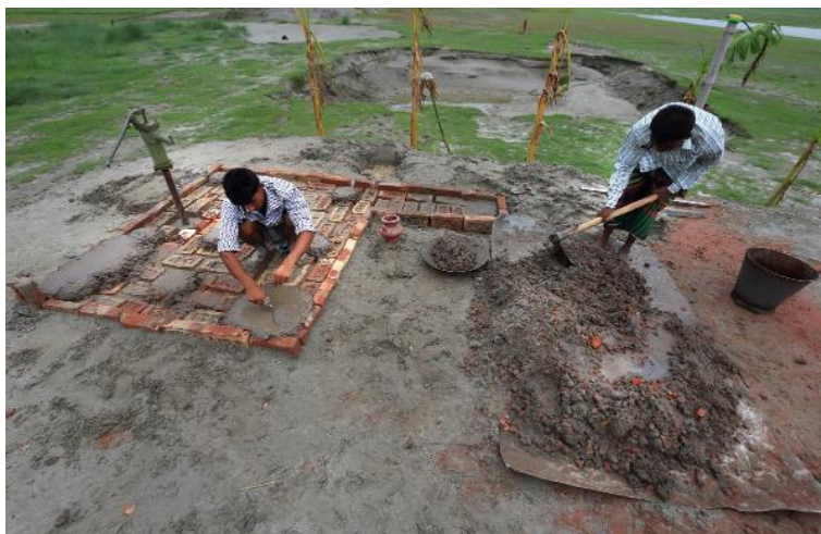
Workers finishing off the concrete platform on a tube well. The platform stops water seeping back down into the well and contaminating it.
