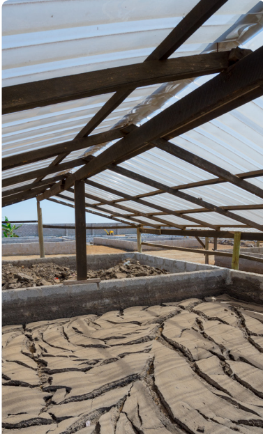
The solids portion of the sludge is transported to drying beds for treatment
