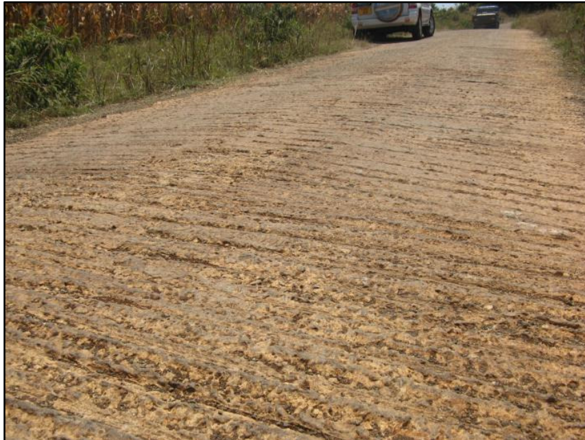
Photo 7: Excessive Grooving on Concrete Slabs (L-K)
