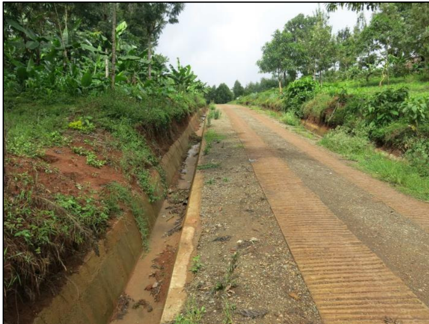
Photo 17: Hazardous Drain (though it helps support the shoulder) (L-K)
