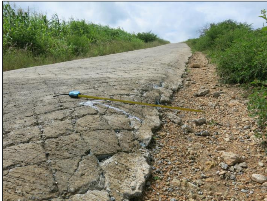
Photo 5: Edge Drop on Concrete Geocells (B-T)
