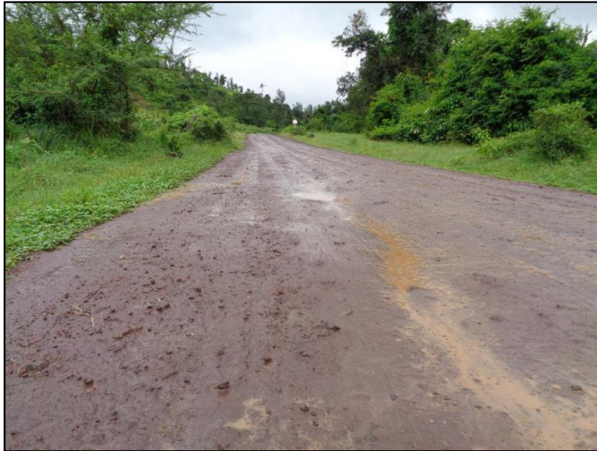
Photo 14: Wet and Slippery Unpaved Surface (L-K)
