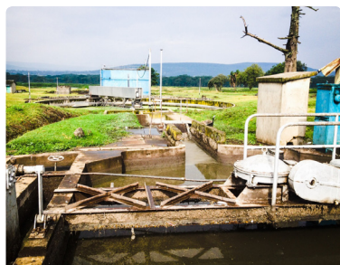
Wastewater treatment facility, Nakuru Photo: Rachel Rose
