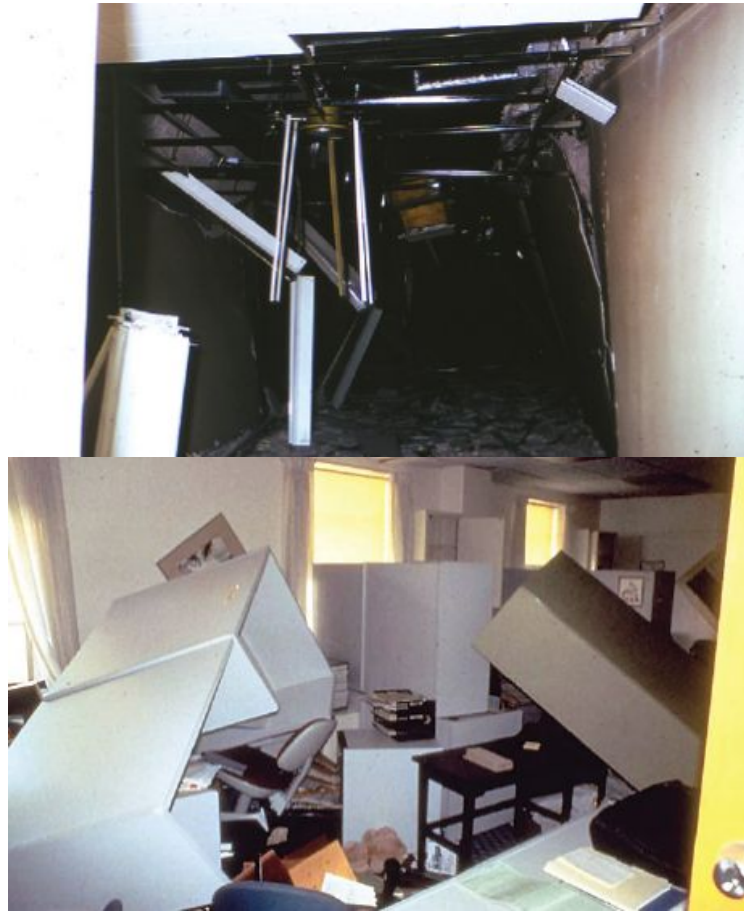
Figure 2 Example of nonstructural damage during an earthquake. Image adapted from FEMA 577 (FEMA, 2007).
