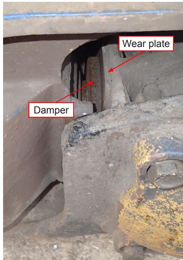
Figure 15: Visibility of the wear plate with the suspension fully assembled
