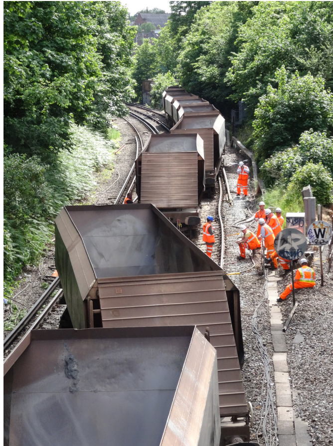
Figure 2: Derailed portion of the train (courtesy of Network Rail)
