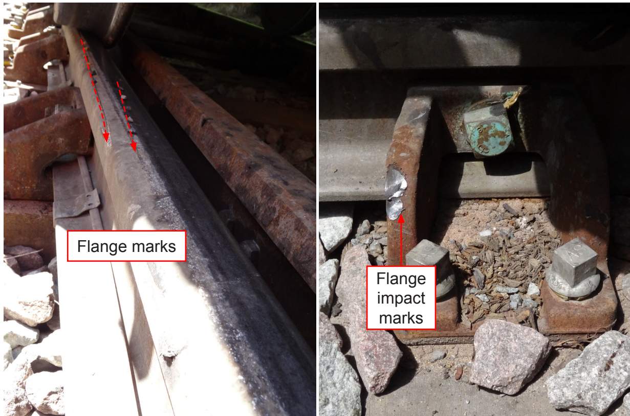
Figure 7: Derailment marks on the rail head and on the subsequent chairs
