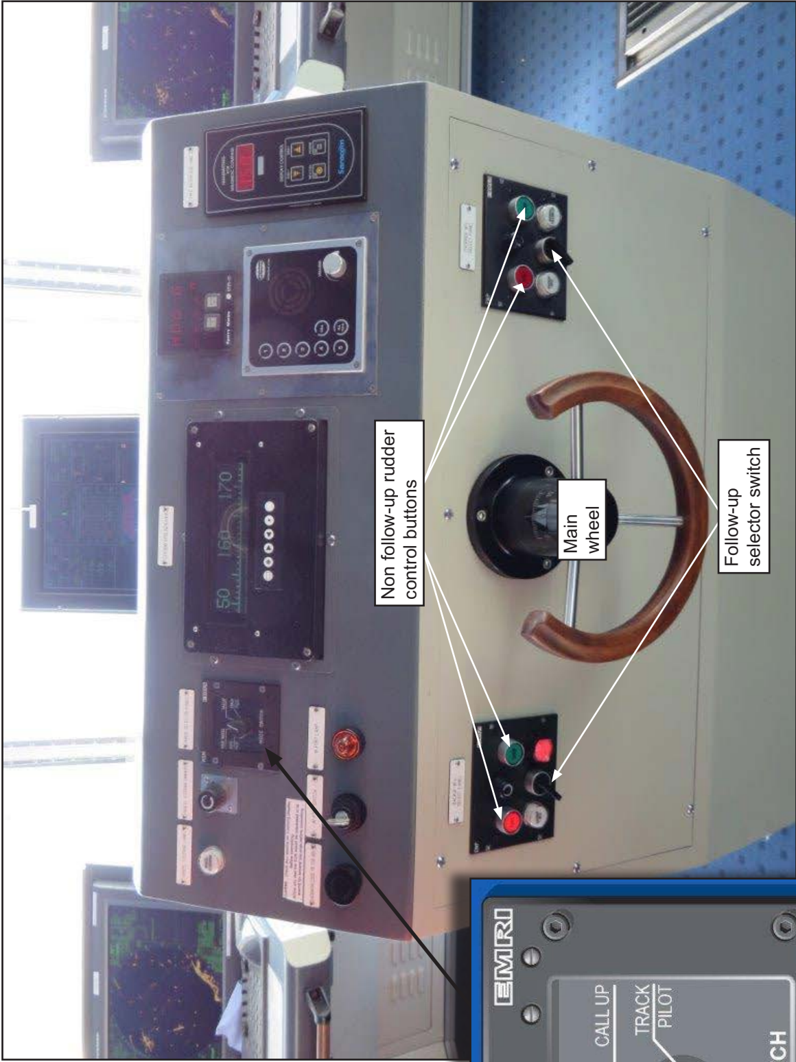
Figure 7: Main steering stand with mode control switch
